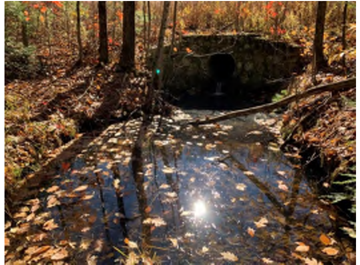
Photo 22. The outlet of Crossing 6 SB 1287+40 is perched, and a large scour pool has formed downstream of the outlet.
