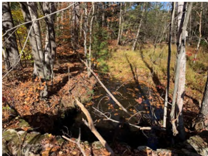
Photo 23. A view of the downstream conditions taken from above the outlet of Crossing 6 SB 1287+40.
