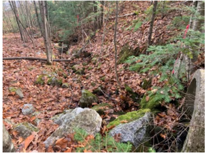
Photo 2. The downstream reach from the outlet of Crossing 4 SB 1198+00 is very steep (~28%) and is strewn with boulders.
