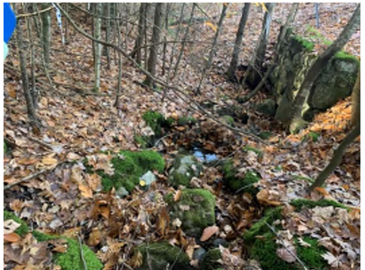
Photo 4. The view facing downstream along the watercourse towards the inlet of Crossing 4 SB 1198+00.
