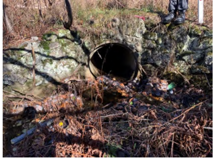
Photo 30. The inlet at Crossing 6 NB 1290+00. The culvert is a 36" reinforced concrete pipe.
