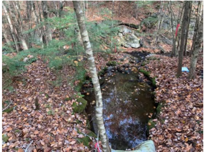
Photo 10. The watercourse carried by Crossing 4 NB 1199+75 free falls over a steep bank and discharges to Stevens Brook.
