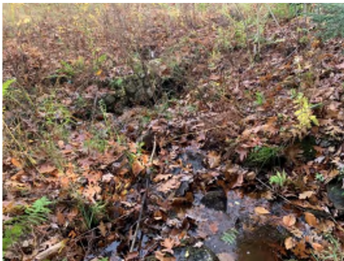
Photo 11. The inlet of Crossing 4 NB 1199+75 was obstructed by leaf litter and other organic debris.
