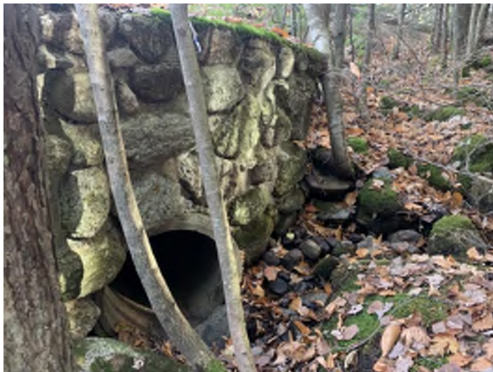
Photo 3. The watercourse takes a sharp bend to enter the inlet of Crossing 4 SB 1198+00.
