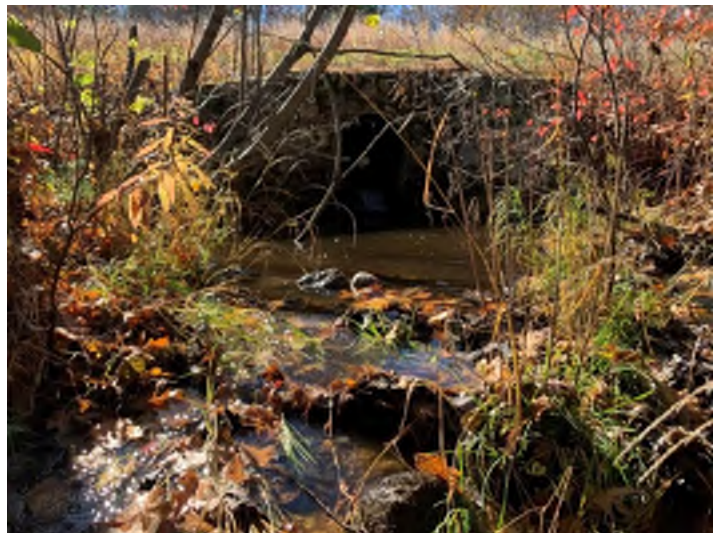
Photo 28. A natural cobble bar/weir within the scour pool at the outlet of Crossing 6 NB 1290+00.
