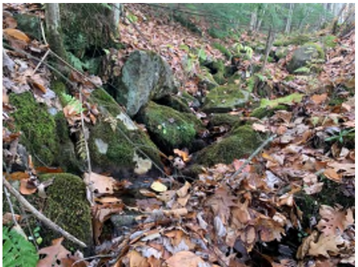
Photo 12. The upstream reach from the inlet of Crossing 4 NB 1199+75 is very steep and strewn with boulders.
