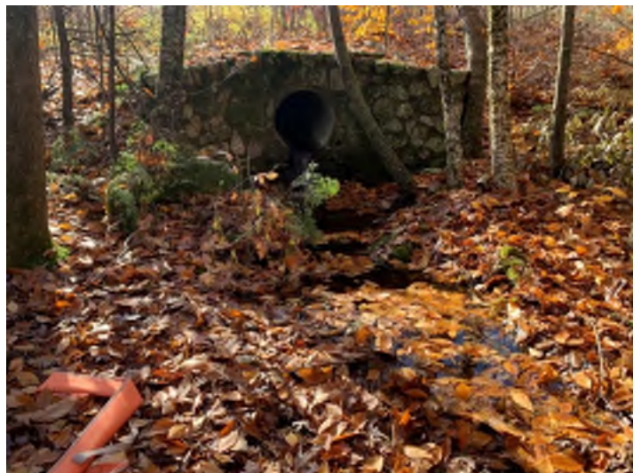
Photo 16. The outlet of Crossing 5 SB 1282+60 is perched by 2 feet. A scour pool has also formed downstream of the outlet.
