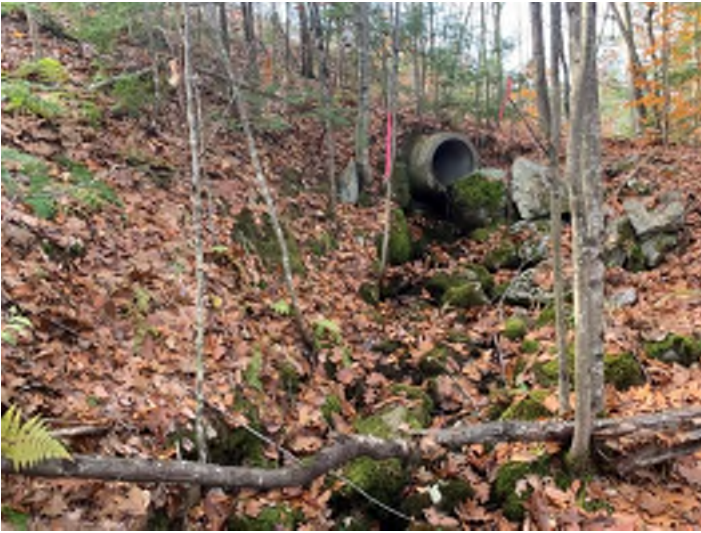
Photo 1. The outlet of Crossing 4 SB 1198+00 is perched.
