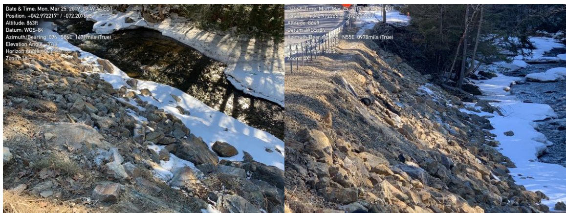
Figure 5-1 Erosion Prevention Along NH 9 in Roxbury
