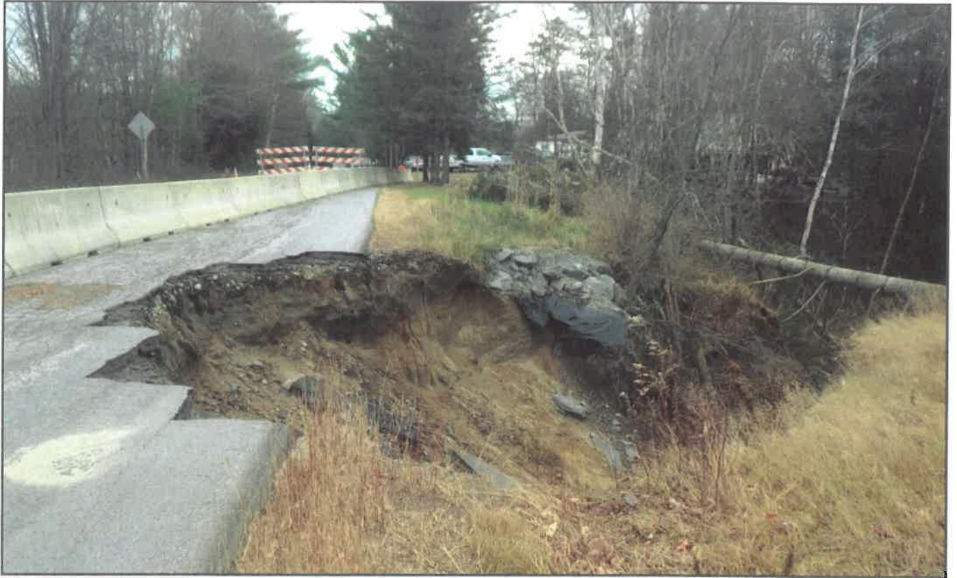
Photo 3: Looking SE at top of slope and road failure
