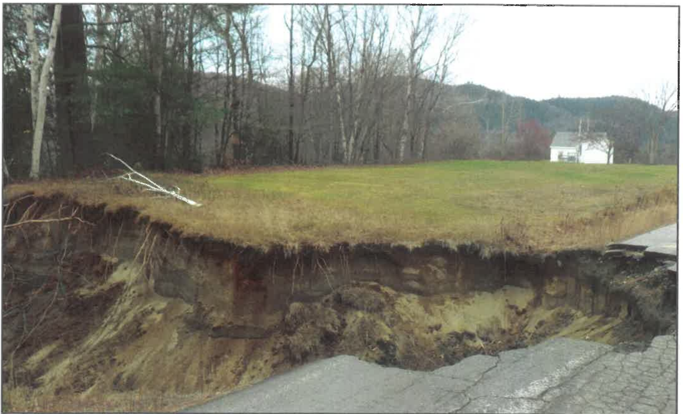
Photo 4: Looking NW at top of slope and road failure
