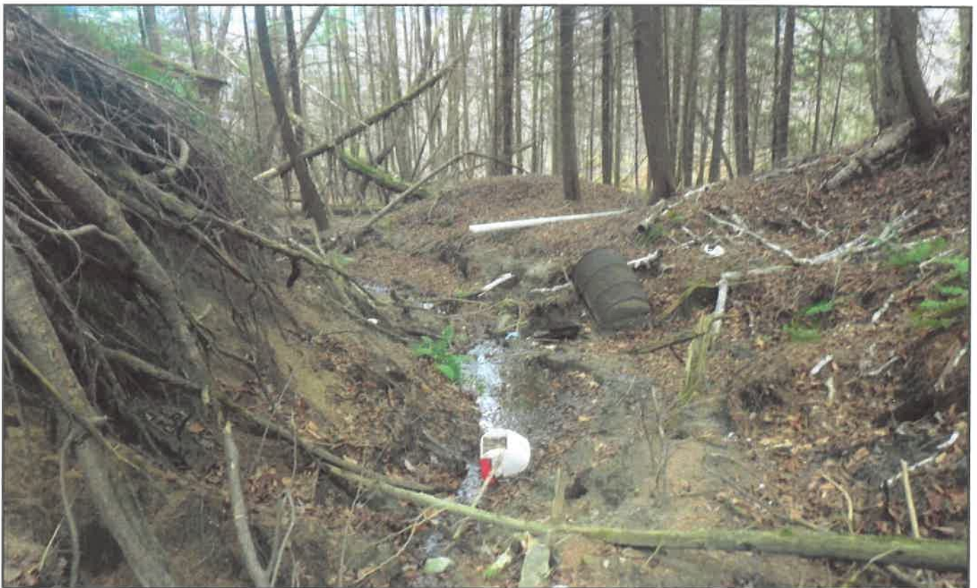
Photo 8: Looking South from bottom of failure
