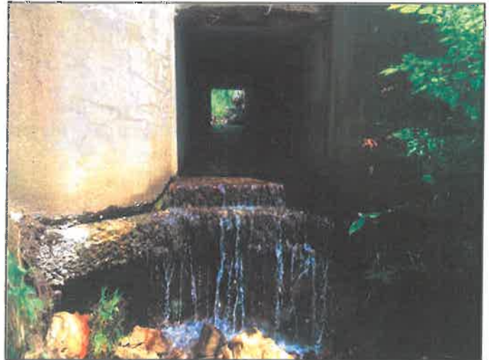
View looking at the perched outlet of the existing crossing structure, which was installed in 1938. The structure is a complete barrier to upstream aquatic organism passage.
