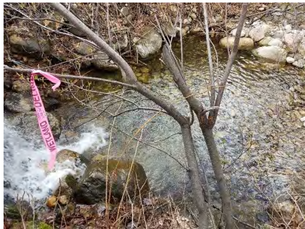
Photo 15: Scour pool at the outlet. Approximately 18' long and 15' wide.
