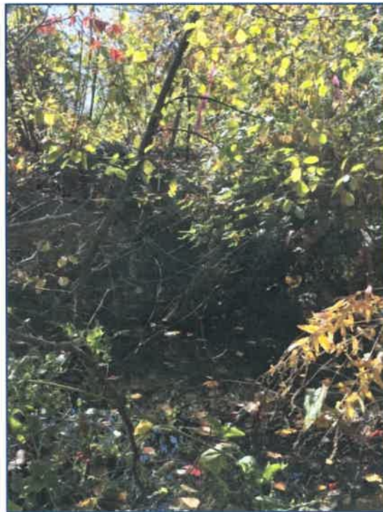
Photo 6- View south toward new driveway (built 2008). Twin 24" plastic culverts (to be replaced and lowered) are partially obscured by vegetation. Wetland area A2 in foreground.
