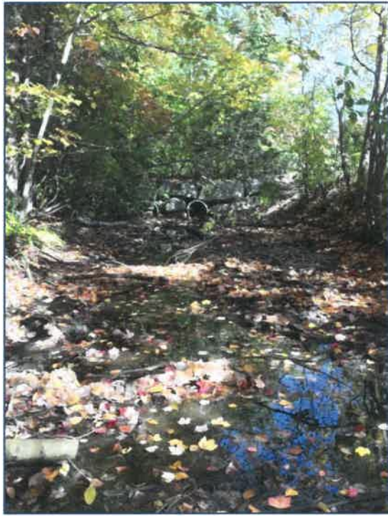
Photo 7- View north along Wetland area A2 (excavated drainage ditch) toward old driveway (built in 2003, to be removed). Twin 21" plastic culverts and stone header clearly visible.
