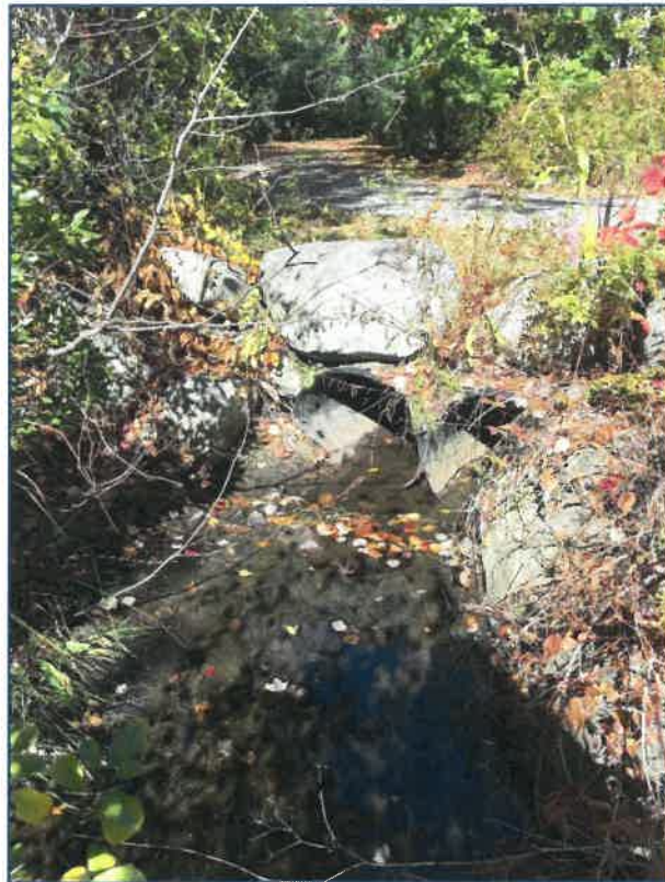
Photo 4- Closeup (looking north) of new driveway (built 2008) with stone header and twin 24" plastic culverts shown. Standing water in Wetland area A1.
