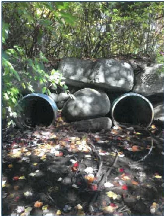
Photo 8- Closeup of old driveway (built 2003, to be removed). Twin 21" plastic culverts also to be removed. Note overgrown vegetation atop abandoned driveway.
