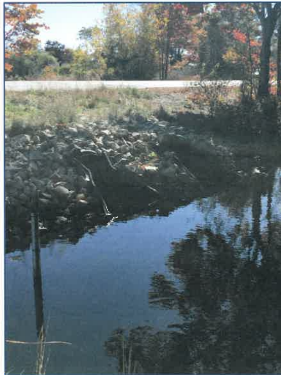
Photo 14- View east along Wetland area A3. Riprap and twin 36" HDPE culvert inverts clearly visible under Route 1A.
