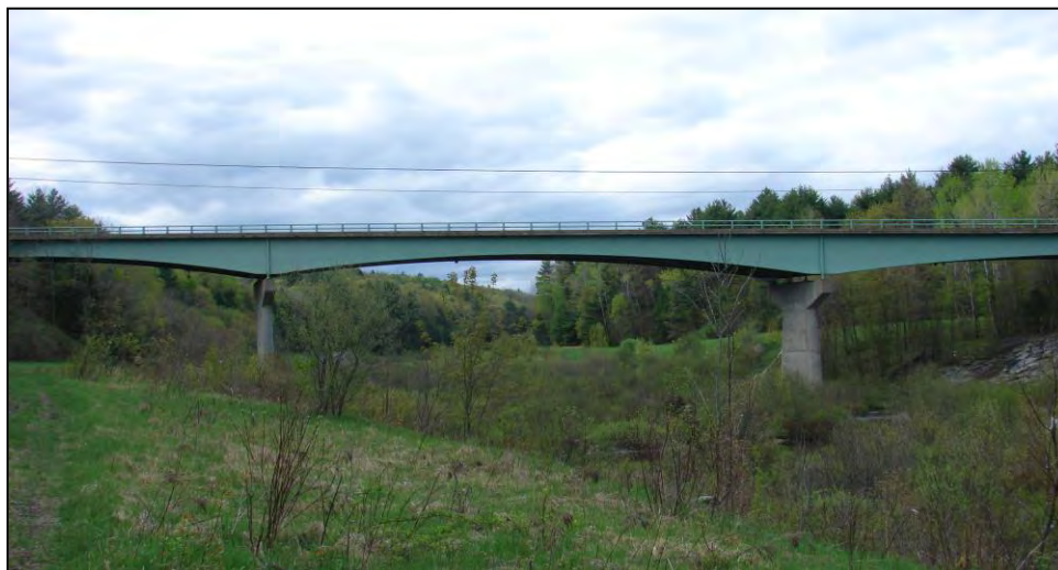
Figure 11. Canal No. 2 Bridge on N.H. Route 77 in Weare (Photograph taken by Patrick Harshbarger).
