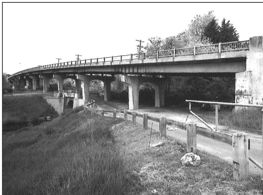
Figure 5: Atkinson Depot Bridge (Bridge No. 105/030), Plaistow (NHDOT, Historic American Engineering Record Documentation).
