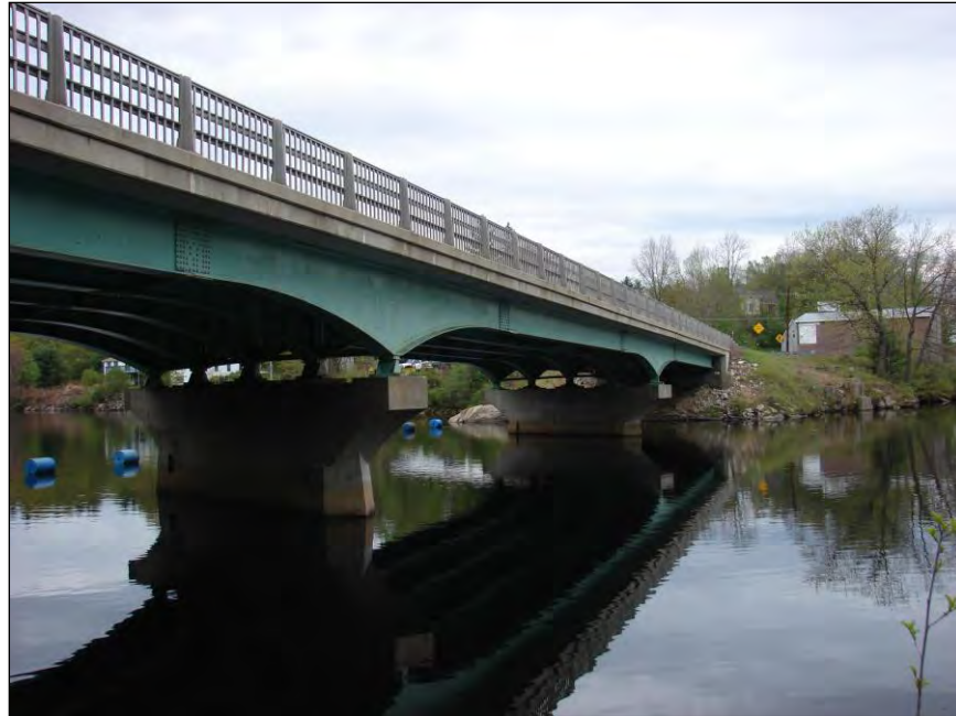
Figure 9. Tremont Street over the Contoocook River in Boscawen. State Bridge No. 131/035 (Photograph taken by Patrick Harshbarger).
