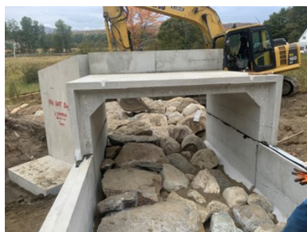
The invert of the box culvert contains flat stones for the wildlife shelf and round stones with gravel infill for stream simulation.
