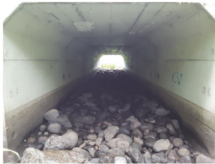
An embedded culvert in Londonderry, NH, that is hyporheic (movement of stream water into the subsurface).
