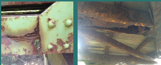
Rust Holes in Steel Members
