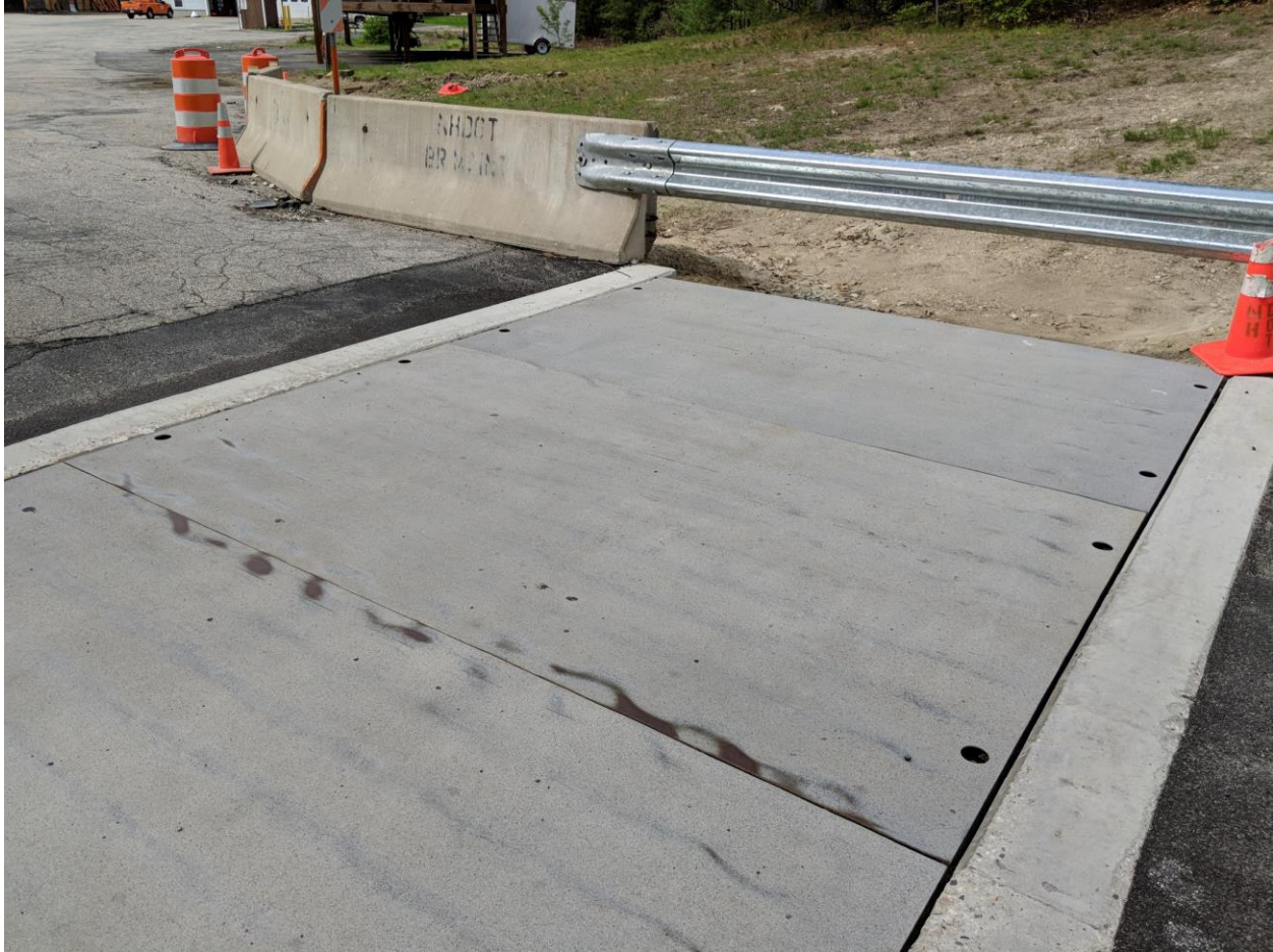
Figure 4: Bridge panels after trafficking showing abrasion and removal of high friction treatment.
