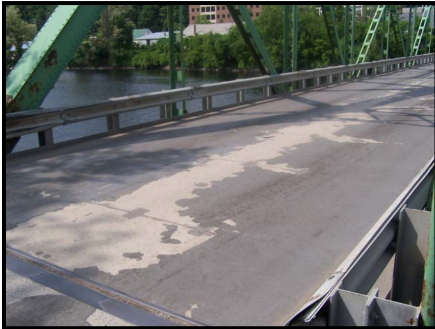
Figure 11 - Failed Stirling Lloyd overlay
