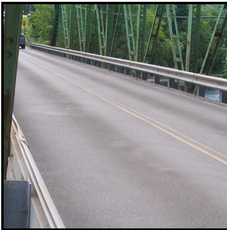
Figure 9 – Flexogrid aggregate wear in wheel path
