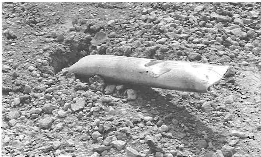
Figure 51 . Single 4 in. aluminum sign support installation anchored in strong soil after test 405231-7.
