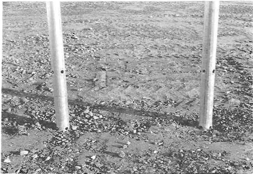
Figure 148 . Dual 4-in with 1-in holes aluminum sign support installation anchored in strong soil before test 405231-23.
