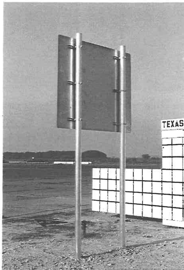
Figure 37 . Dual 4 in. aluminum sign support installation anchored in strong soil before test 405231-5.
