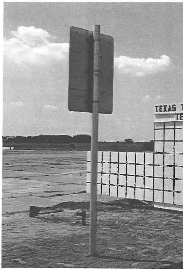
Figure 62 . Single 4 in. aluminum sign support installation anchored in weak soil before test 405231-9.
