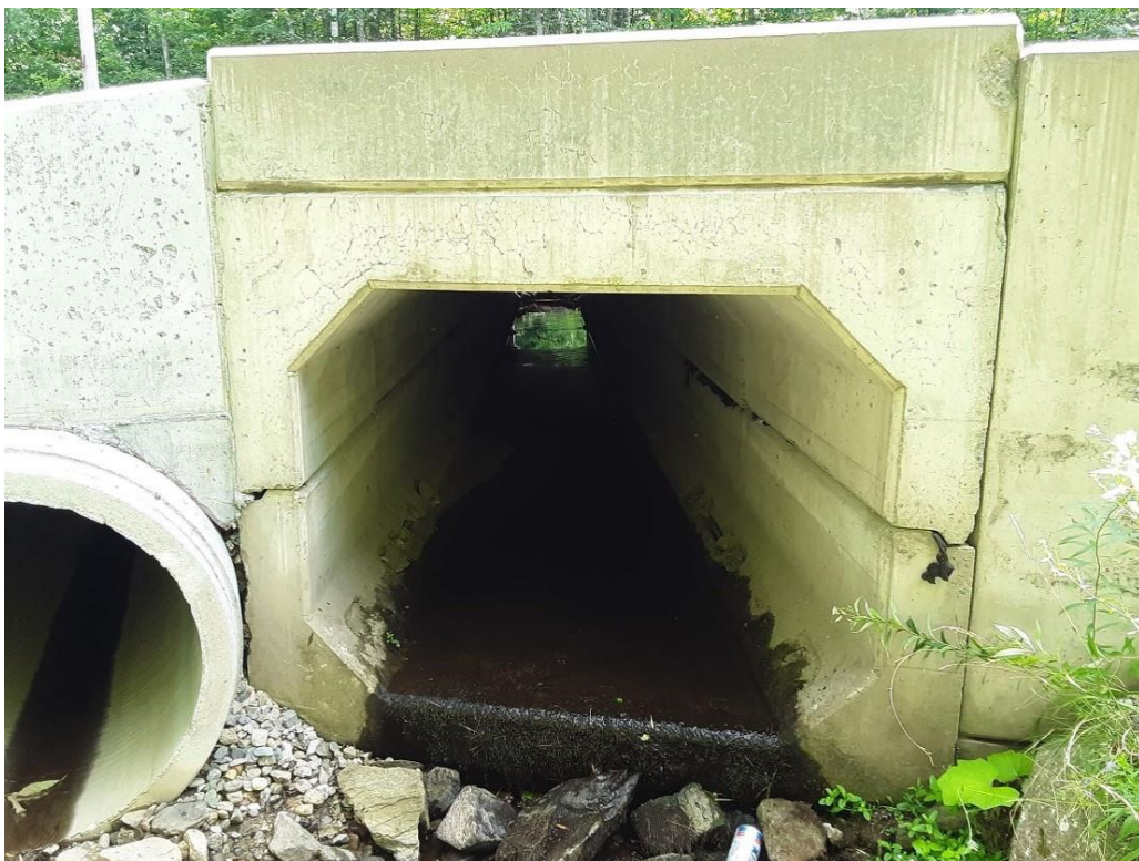
Figure 6: Outlet of Bethlehem Culvert, loss of bed material
