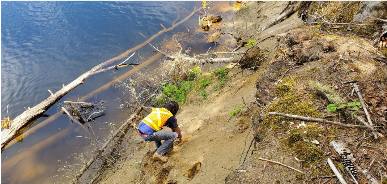
Figure 17. High bank height and steep slope at State Line streambank
