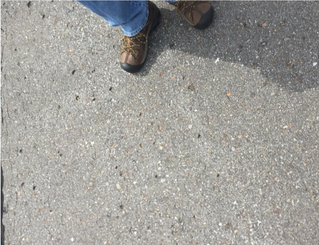
Figure 5: Loss of Aggregate in Runway Surface
