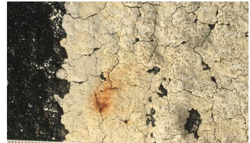
Figure 32: Rust Spot Stain in Area G
