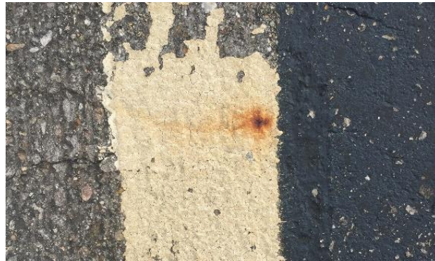
Figure 17: Bottom-up Rust Spot Stain
