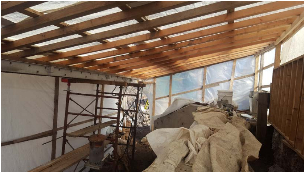
Figure 8: A heated enclosure constructed over a bridge to prevent concrete from freezing during curing.
