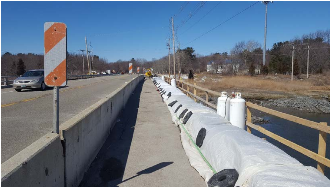
Figure 7: Insulated wrap and heaters on a bridge curb after cold weather placement.
