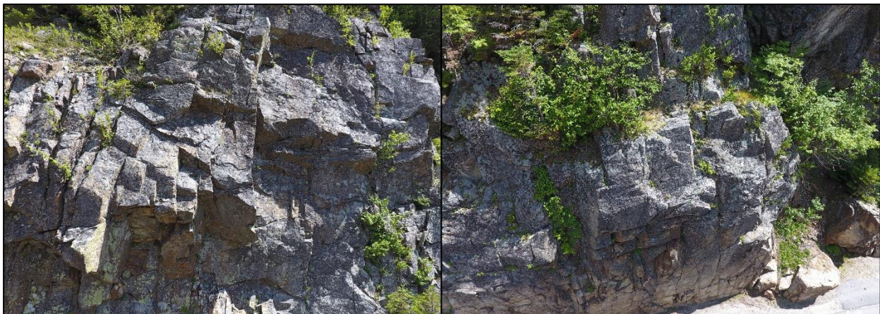
Figure 41. High-resolution inspection photos captured during this case study.
