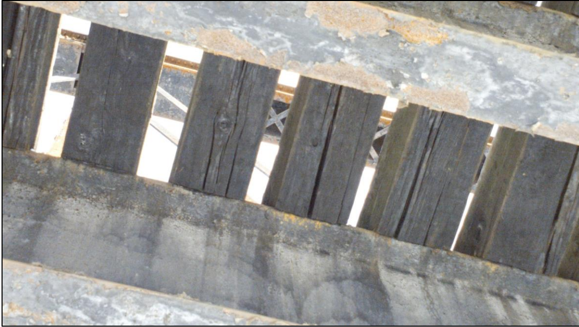
Figure 9. Inspection photo of the underside of a railroad bridge captured by the senseFly Albris.
