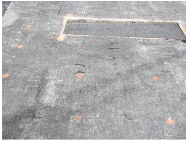
cracks caused by poor anode cover
