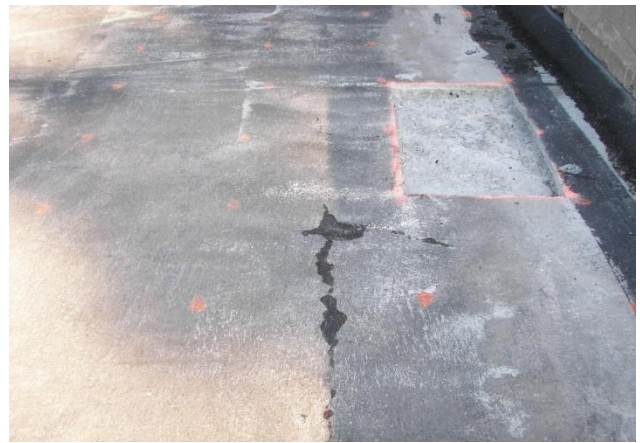
longitudinal cracks at mid deck
