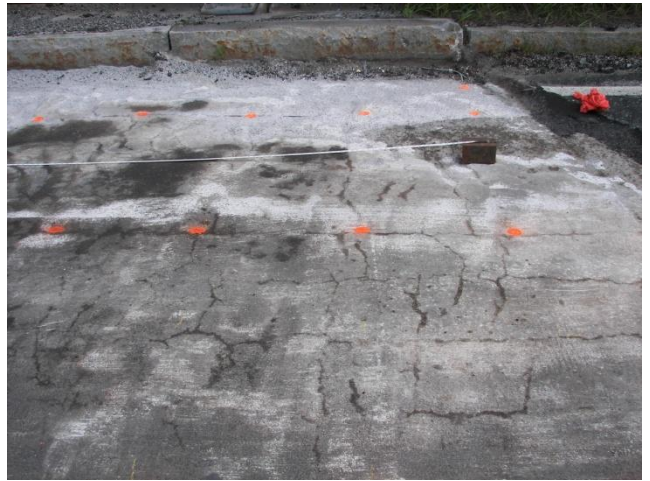
close-up of cracks
