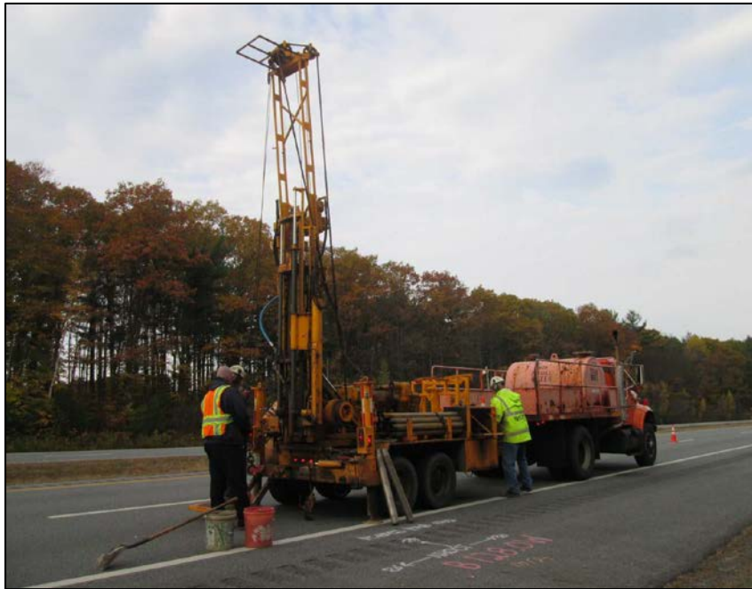
Figure 10. Test section drill rig setup at WB MM 128.0 for core hole sampling and geotechnical soil sampling.
