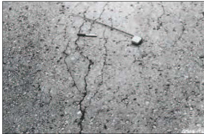
Figure 1. An example of fatigue cracking in flexible pavement (DOD 2001).
