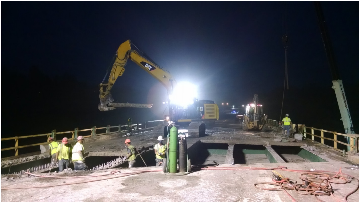
Figure 12 - Slab removal with haunch concrete demolition and shear connector removal in progress.
