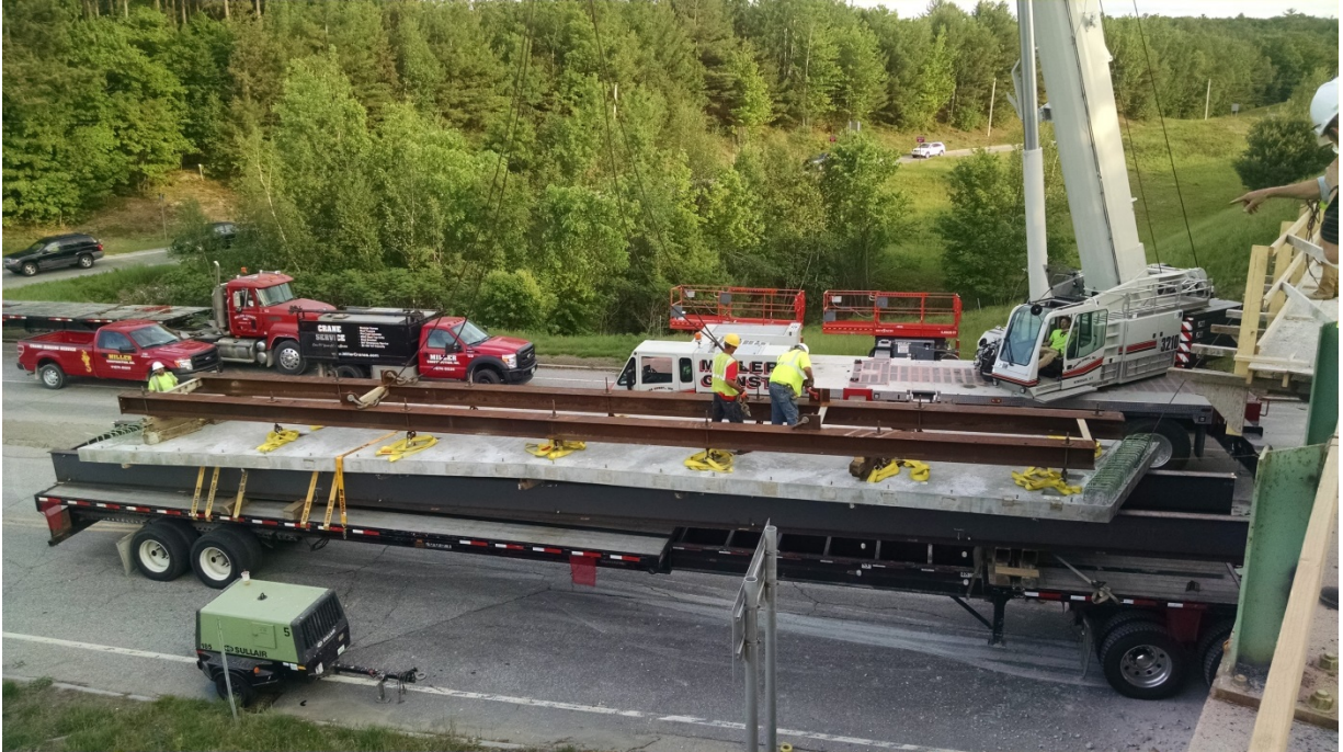
Figure 17 - Panel on shipping frame (bottom) with lifting frame (top) prior to erection.
