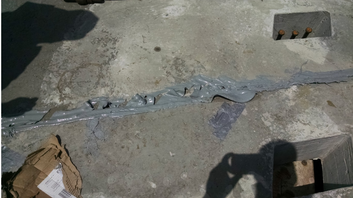
Figure 25 - Apparent joint failure with large surface deformation and polymer break-up.
