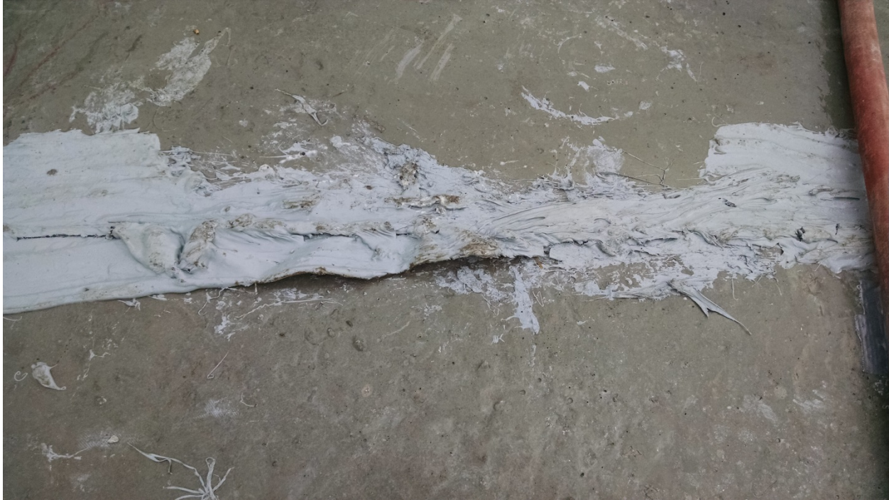
Figure 24 - Polymer delamination due to continued deflection.
