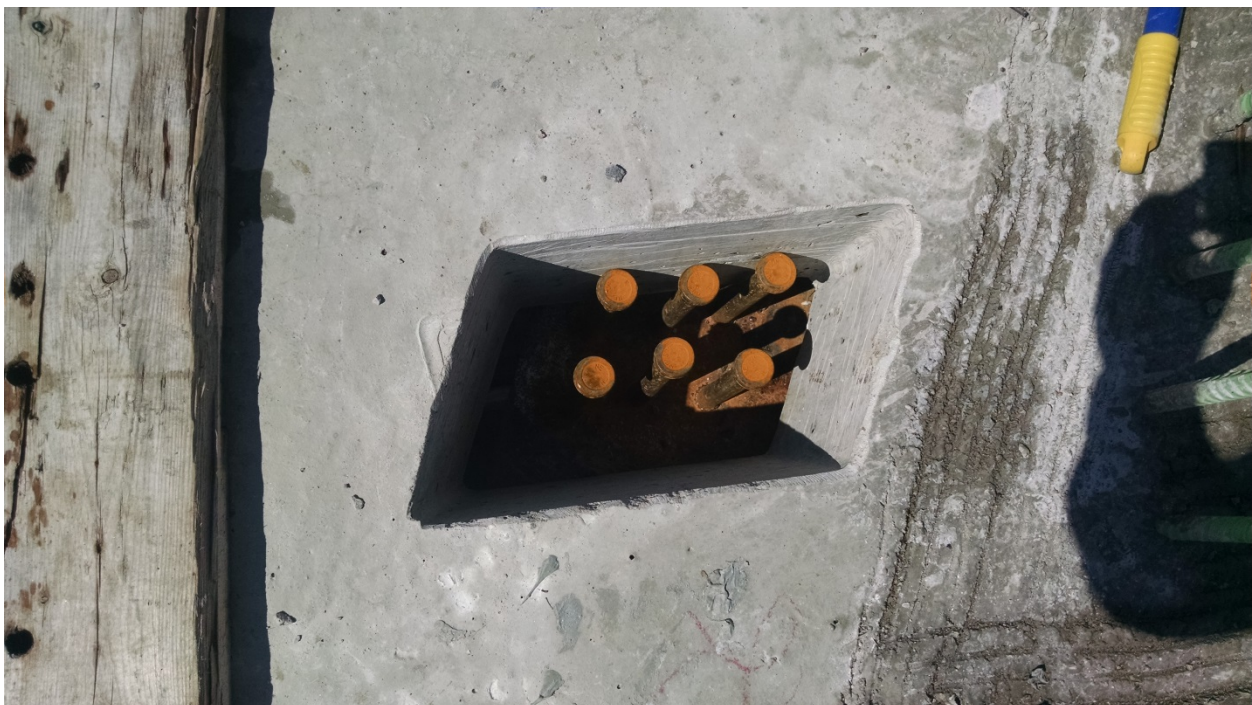
Figure 27 - Shear connector group after apparent girder expansion prior to grouting.
