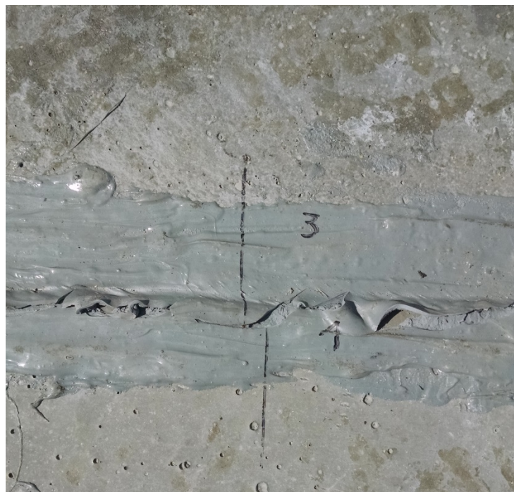
Figure 26 - Apparent failure of the Panels 3 and 4 joint (3:20pm 6/6/16).
