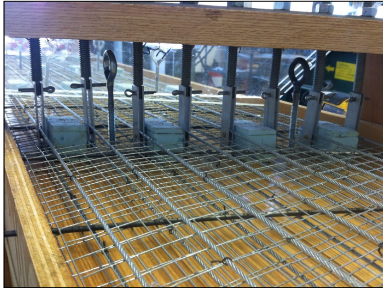
Figure 11: Prestressing Cables at Crown
