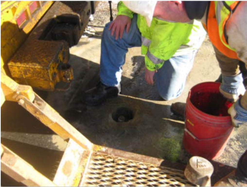
Figure 10. Frost-tube installation, backfilling with the PVC pipe covered to prevent clogging the pipe.
