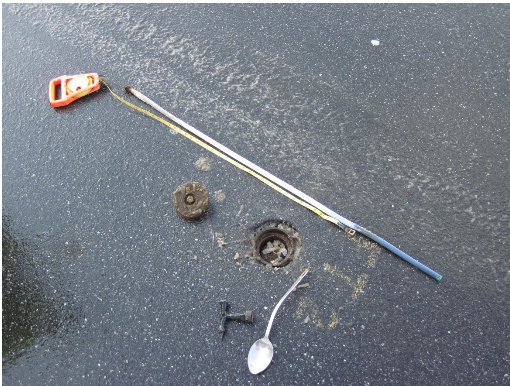
Figure 11. The method of measuring the frost and thaw depth with the frost tube at FT2 on 2 March 2015. The depth from the pavement surface to the top of the tube at this location ranged from 2 to 3 in. Frost-depth measurements provided in Fig. 12 and 13 reflected this dimension.
