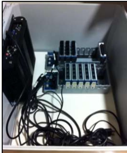
Figure D-9: Photograph of Enclosure and DAQ Equipment
