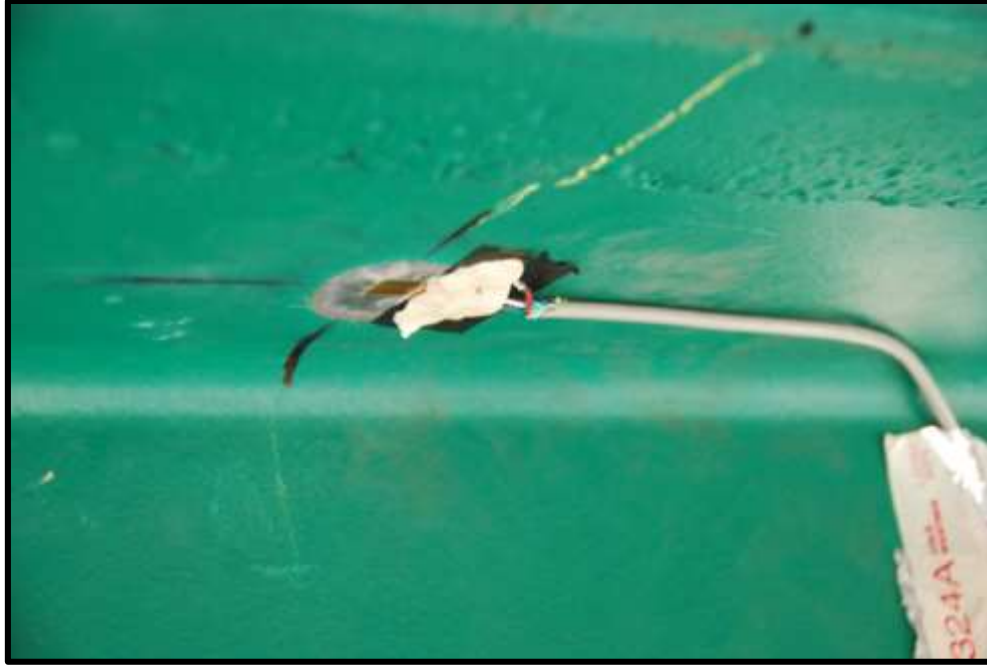
Figure G-3: Photograph of Full Bridge Strain Gauge Installed on the Top Flange of Beam D, South Face
