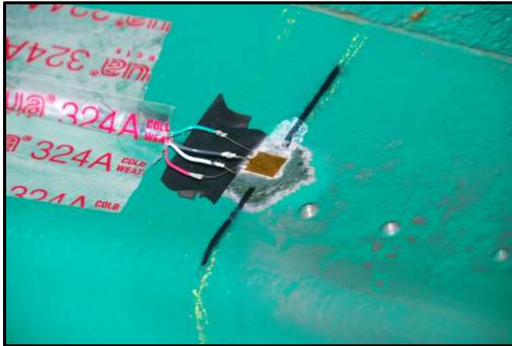
Figure G-9: Photograph of Full Bridge Strain Gauge on the Top Flange of Beam E, North Face
