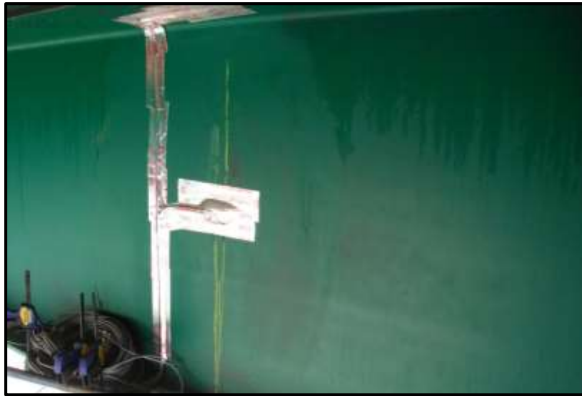
Figure C-22: Photo of Condensation on Beam Surface
