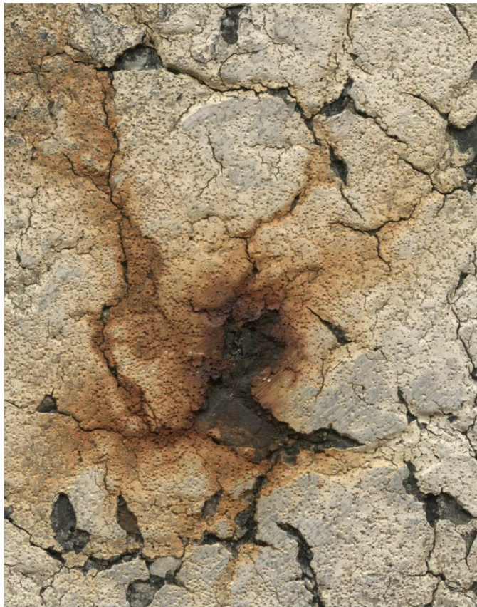
Figure 2 Close up of Figure 1 showing iron staining
