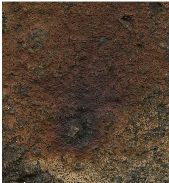
Figure 21 close up of Figure 20 showing major staining
