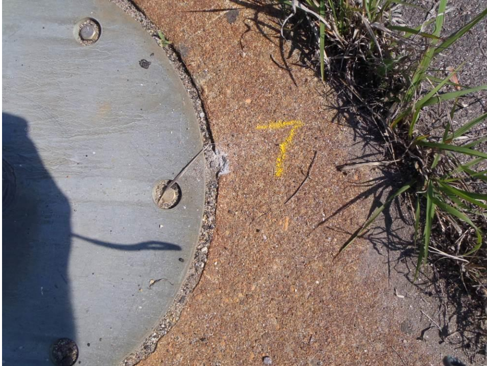
Photo 7 – Close up of paint sample 7 taken on the concrete light bar at the end of Runway 8.
