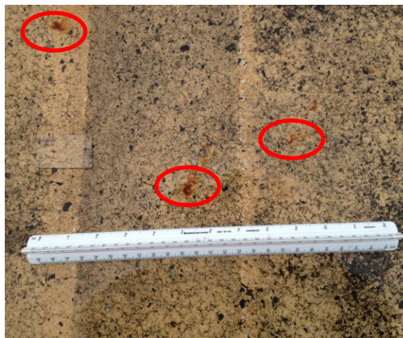
Figure 2–Point stains (red circles)
