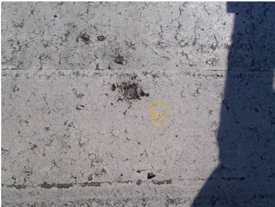
Photo 8 – Close up view of paint sample 8 taken near the centerline of the threshold bar on Runway 8.
