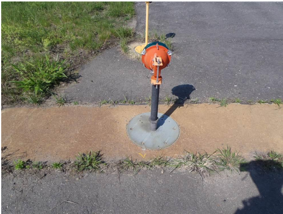
Photo 6 – Southern most runway end light Runway 8. Paint sample 7 taken at base of light.
