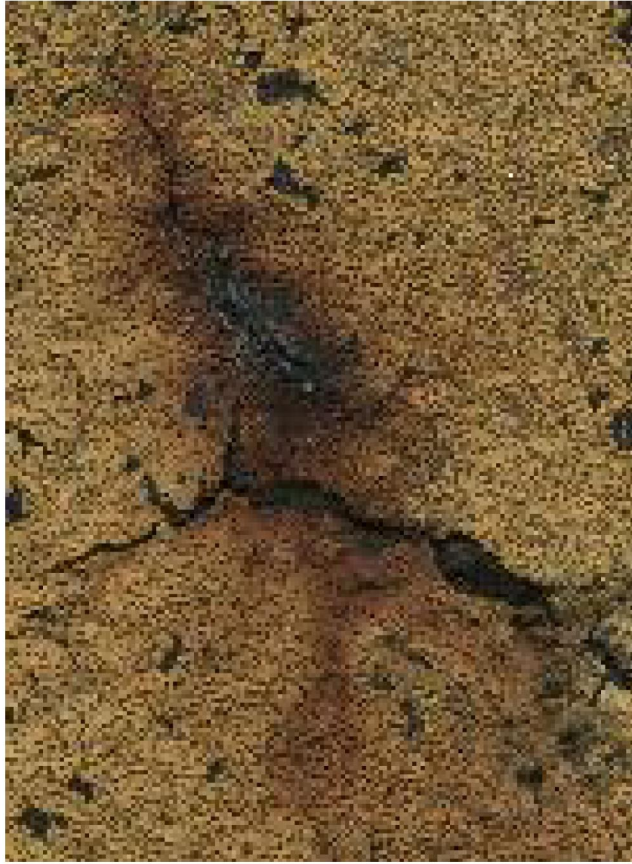
Figure 13 close up of stained area in Figure 12
