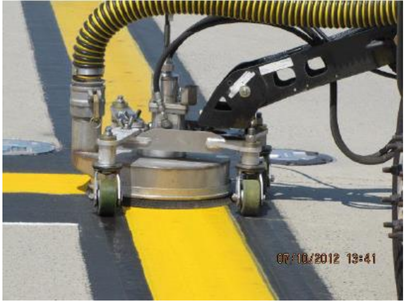
Figure 10 - Paint restoration (Speidel, 2008)
