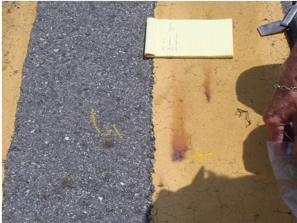
Photo 6 – Paint sample locations 4 & 5 western end of taxiway Hold Line
