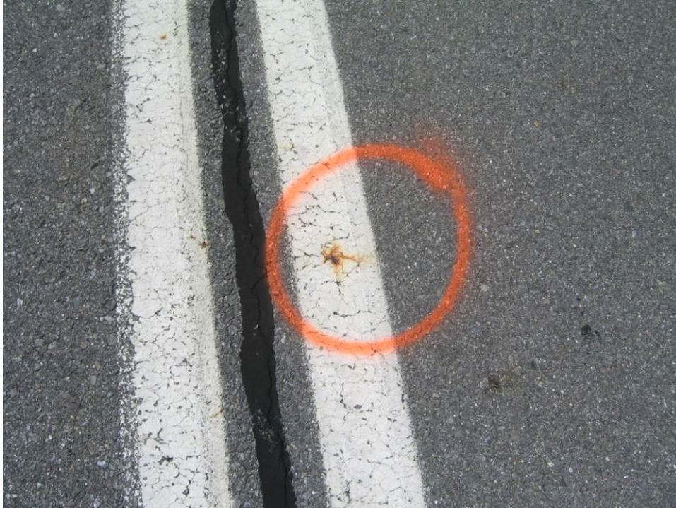
Photo 1 – Close up of paint sample.
