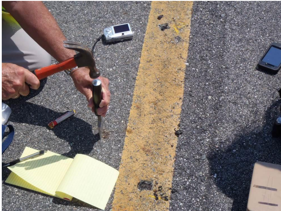
Photo 4 – Sampling of rust stain location 3.
