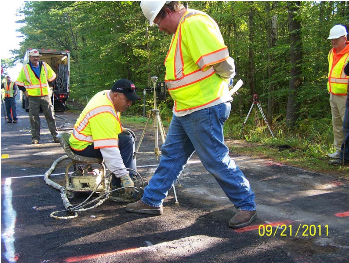
Injection of two-part polymer formulation 1-mm vertical pavement movement measured by laser level
