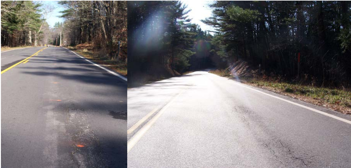
Conditions 1 year after installation: Northbound (left), Southbound (right). Note that inadequate pavement thickness at center of lanes provided marginal structure.
