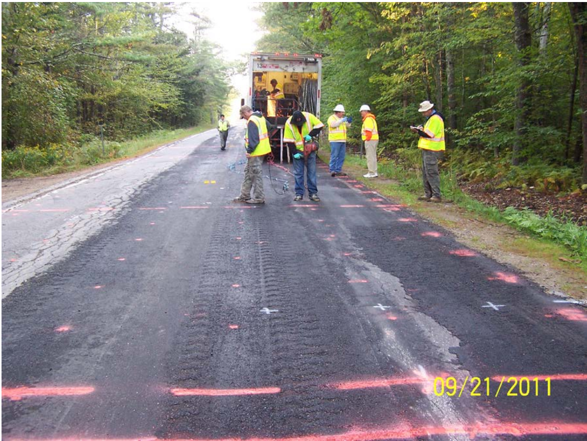
Red paint indicates 4-foot polymer injection grid on HMA shimmed surface Foreground is the southerly transition zone Workers standing in the full treatment area
