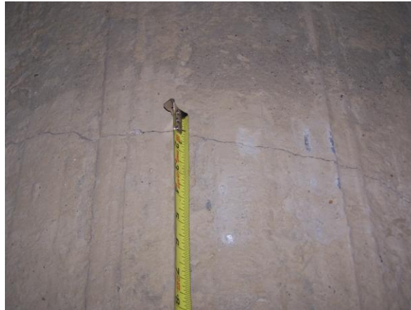
Figure 36: Horizontal crack in secondary pile
