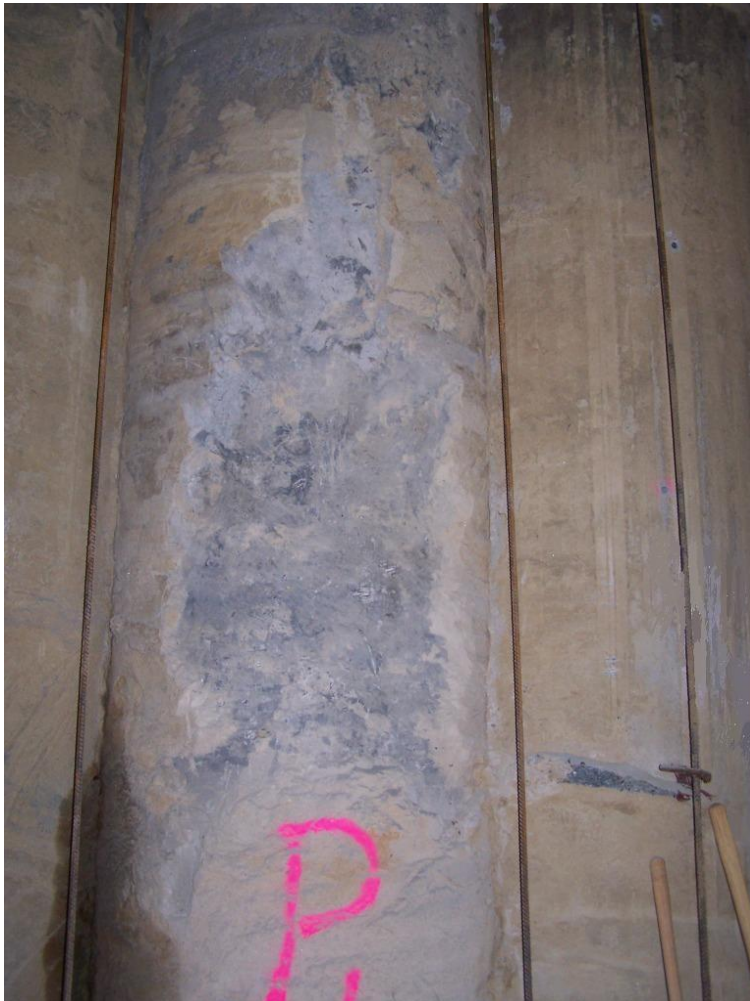
Figure 25: N3P1 chipped down to concrete
