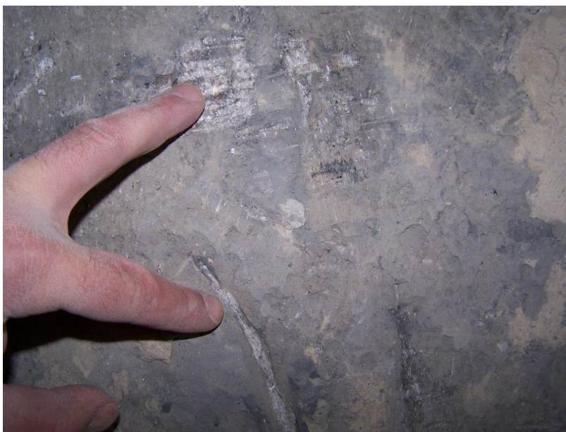
Figure 26: Fingers pointing to slits of exposed light grey concrete on N3P1, darker gray material around concrete is part of the hard layer that formed around the pile
