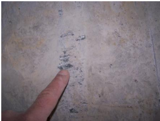
Figure 33: Close up of hammer marks on N3P7
