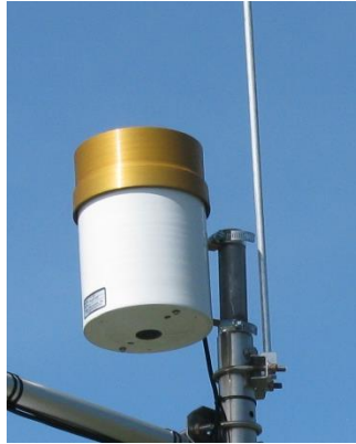
Figure 11: TE525 gage as installed.
