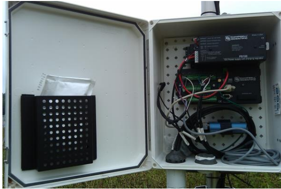
Figure 13: CR1000 and PS100 power supply inside cabinet.
