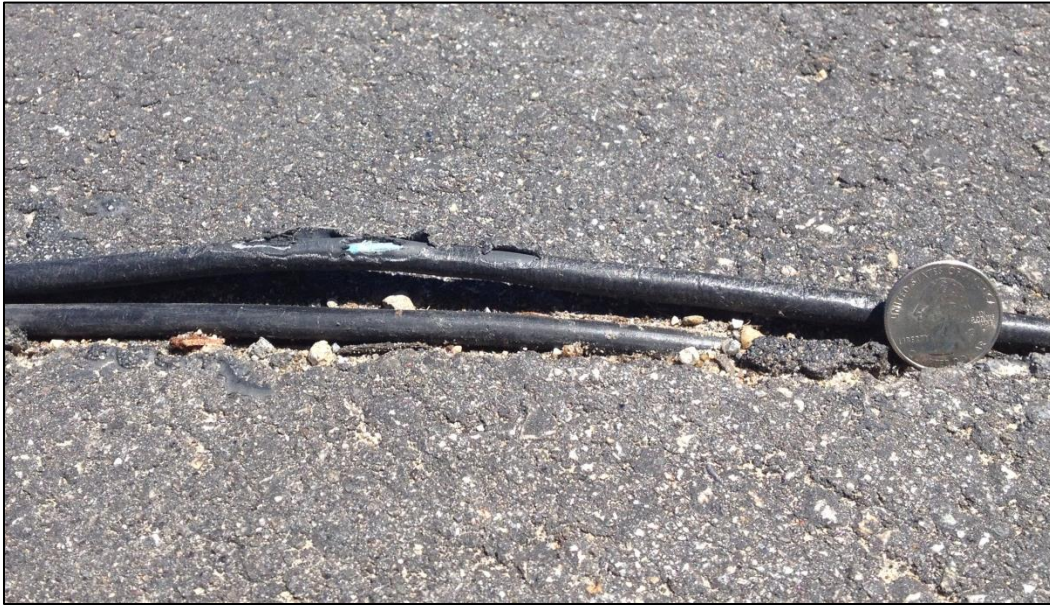
Figure 36: Damaged exposed sensor strip loop wires on the hard shoulder.
