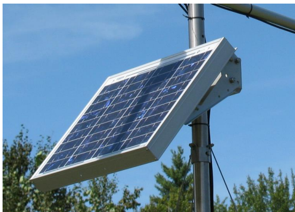
Figure 14: SP20 solar panel installed on weather station.
