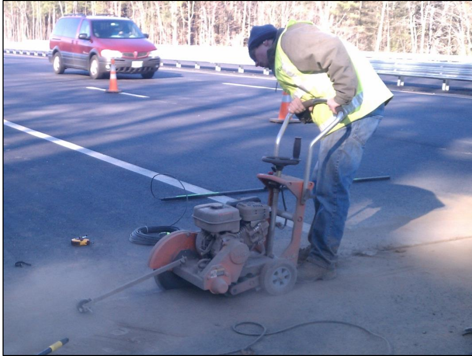
Figure 33: An adjustable-depth pavement saw being used to cut through the wearing course.
