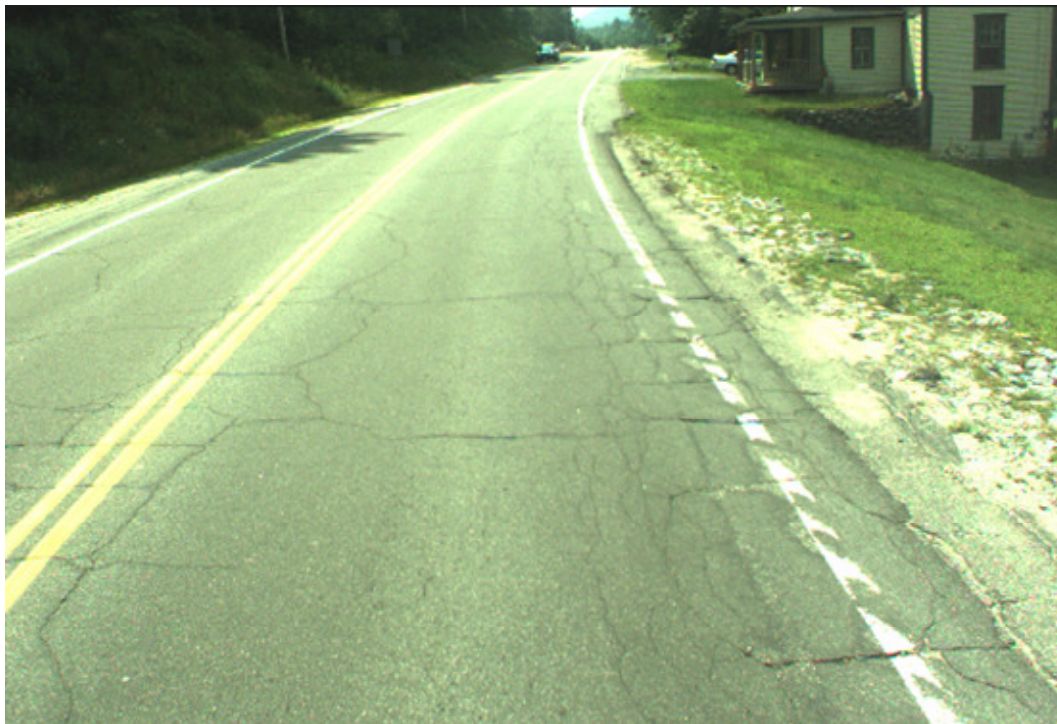
Figure 7. State Route 103 eastbound—A localized weak area resulted in high deflections about 3 miles east of the traffic circle/park.
