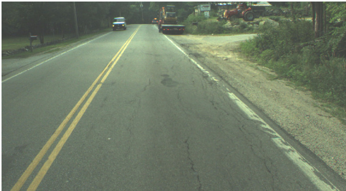
Figure 8. NH 3A southbound—Fatigue cracking in the outer wheel path resulted in high, variable deflections just south of the Bow Maintenance Shed.
