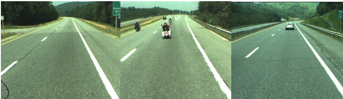
Figure 6. I-89 northbound—(from left to right) A pavement change corresponding to a change in deflections at mile marker 36.4. Lower deflections prior to the pavement change at mile marker 34.6. A distressed area with higher, more variable deflection at mile marker 51.
