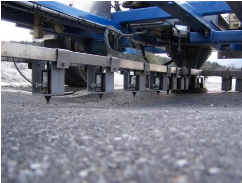
Figure 27 Sensors not touching uneven pavement at Warren Flats
