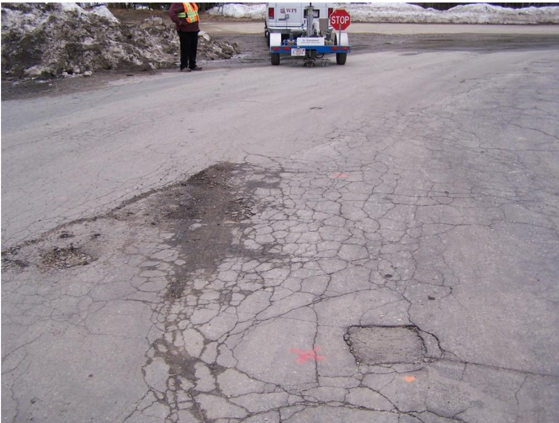
Figure 24 Rumney Site showing the difference in pavement conditions between Stations 6 and 7 in the foreground and Stations 8-10 in the background. The FWD is on Station 10.
