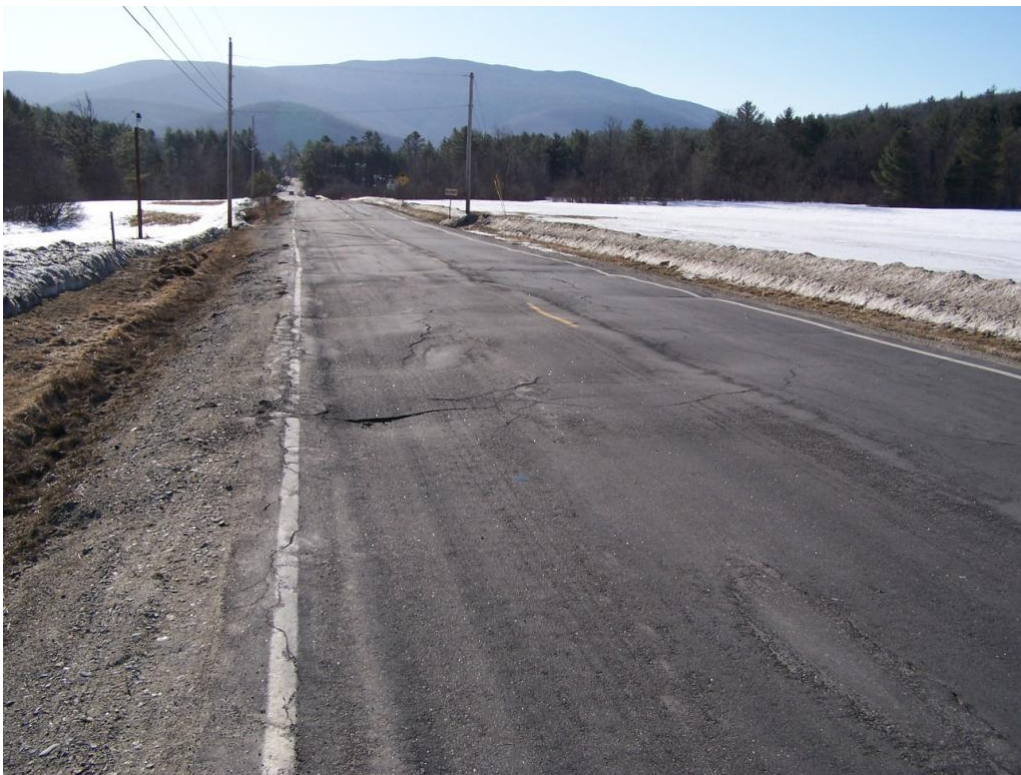
Figure 30 Warren Flats site in the spring of 2009 with heavy reflective cracking through the shim and the same heaving problems
