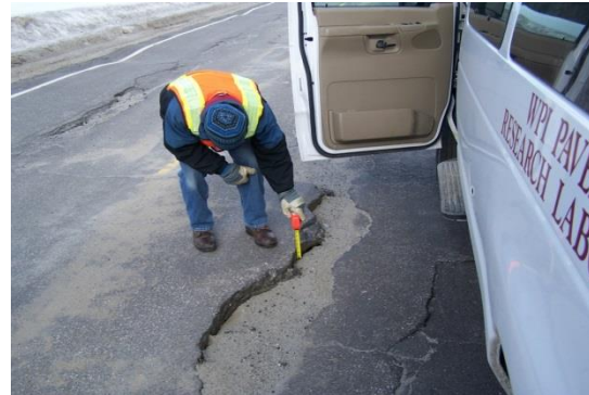
Figure 28 Three-inch differential heaving at Warren Flats
