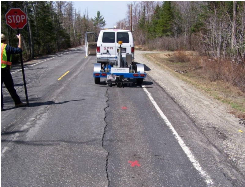
Figure 31 Longitudinal crack at Lake Tarleton running alongside Stations 7 to 10
