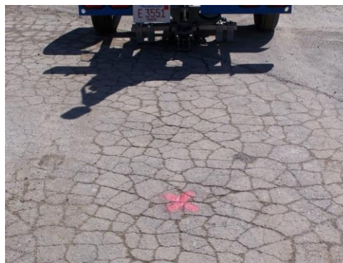
Figure 26 Heavy cracking typical at Wentworth shed site
