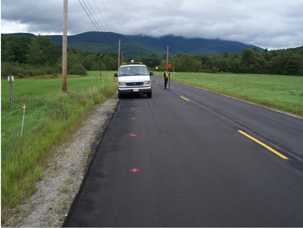
Figure 29 Warren Flats site in August of 2008 shortly after being shimmed
