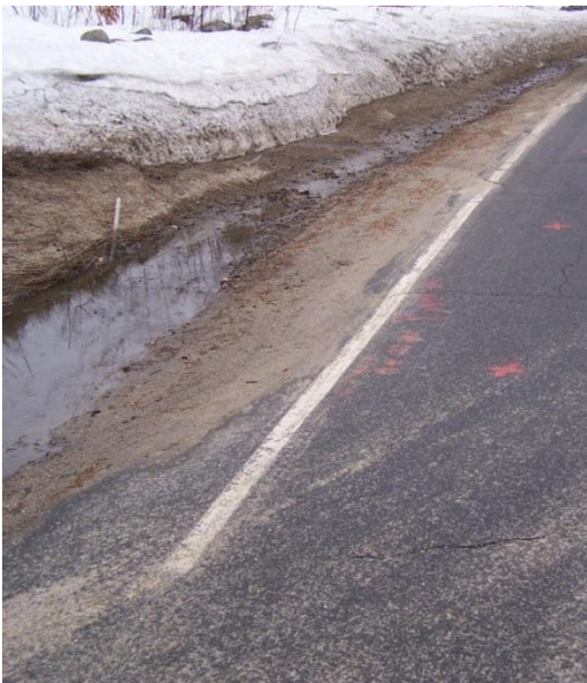
Figure 22 Standing water in ditchline alongside of North Groton Road site in April 2008
