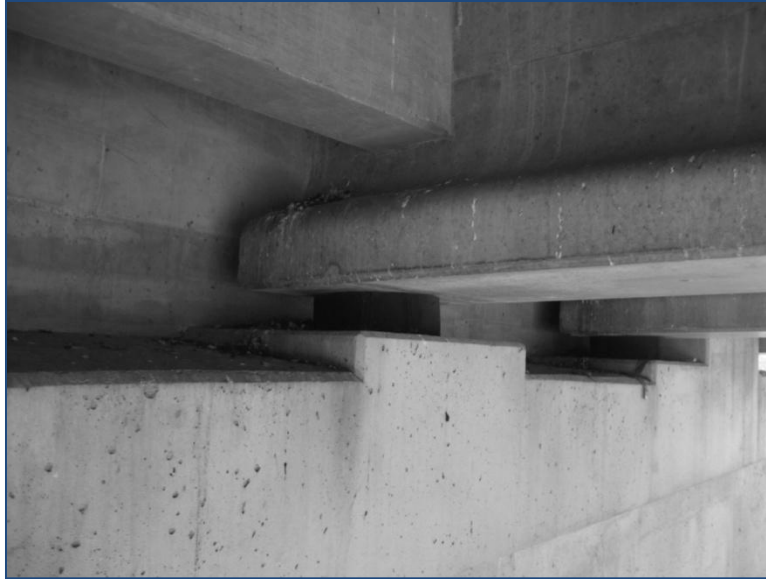
Figure 1: Steel reinforced elastomeric bearing pad at Rollins Road Bridge
