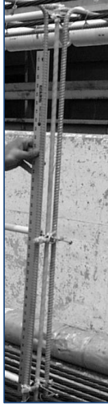
Figure 12: Strain gauges in NEBT girder before prestressing (Adapted from (Bowman M. M., 2002))
