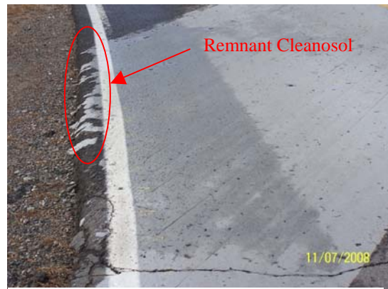
Brown Road, Groveton Edge Wear of Cleanosol (End Strip is Worn Away Due to Lack of Shoulder Material)
