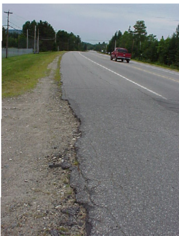
Fig. 1 -- Southbound shoulder edge is broken from stud damage during snowmobile acceleration to cross highway.
