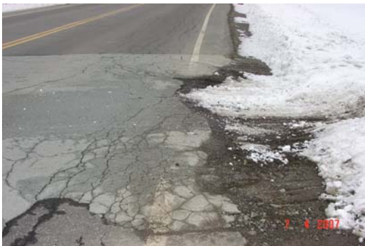
NH Route 26 Shoulder Erosion and Edge Chipping
