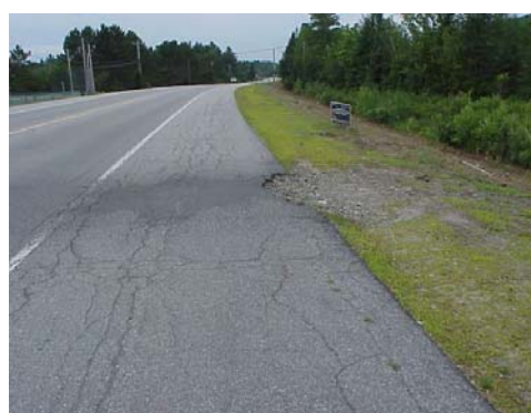
Fig. 2 – Northbound shoulder edge is broken and pavement surface is worn from snowmobile studs.
