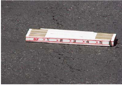
Figure 1 – Cracks along edge of former Rumbles (Section B)
