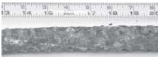
Loss of cross section of rock bolt from corrosion.
