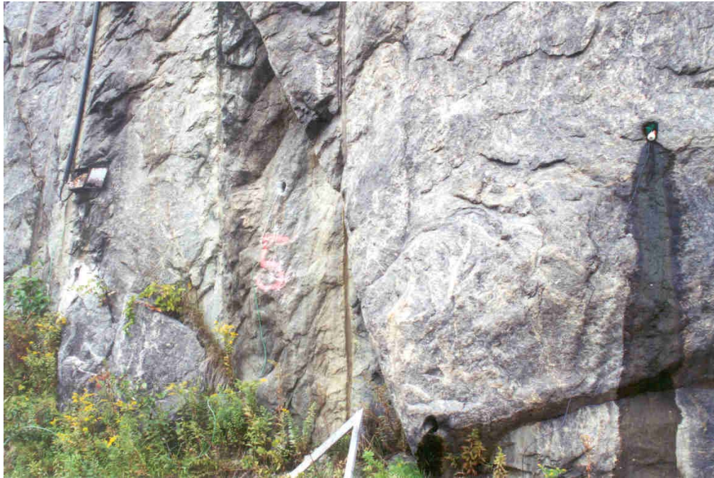
Photograph 5 – Half-cell location for Tendons 5-1 and 5-2. Half-cell is placed in the hole directly above the water stain (right).
