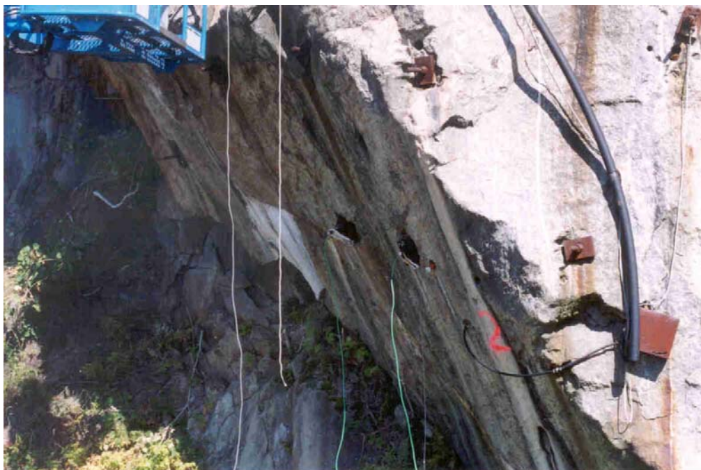
Photograph 7 – Half-cell location for Bolts 1 and 2. Half-cell was placed in a hole to the right of Bolts 1 and 2 (center).
