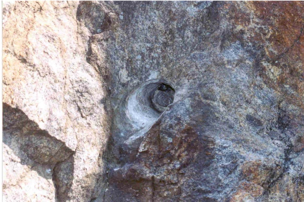
Photograph 5 – Exposed end of Tendon 3-2 after chipping
