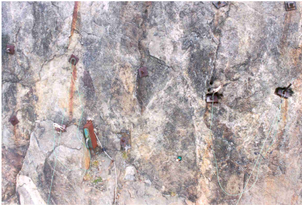
Photograph 10 – Half cell location for Bolts 11 and 12. Half-cell was placed in a hole between and below Bolts 11 and 12 (lower center).
