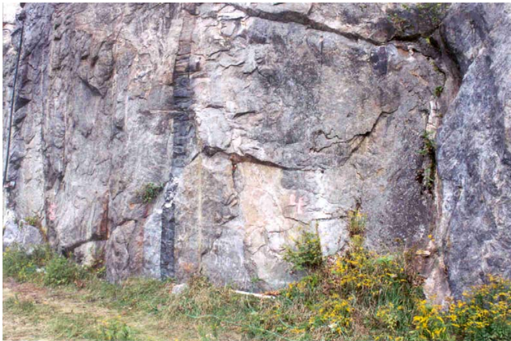
Photograph 4 – Half-cell location for Tendons 4-1 and 4-2. Half-cell is located at the intersection of the vertical and horizontal crevices in the center of the photograph.
