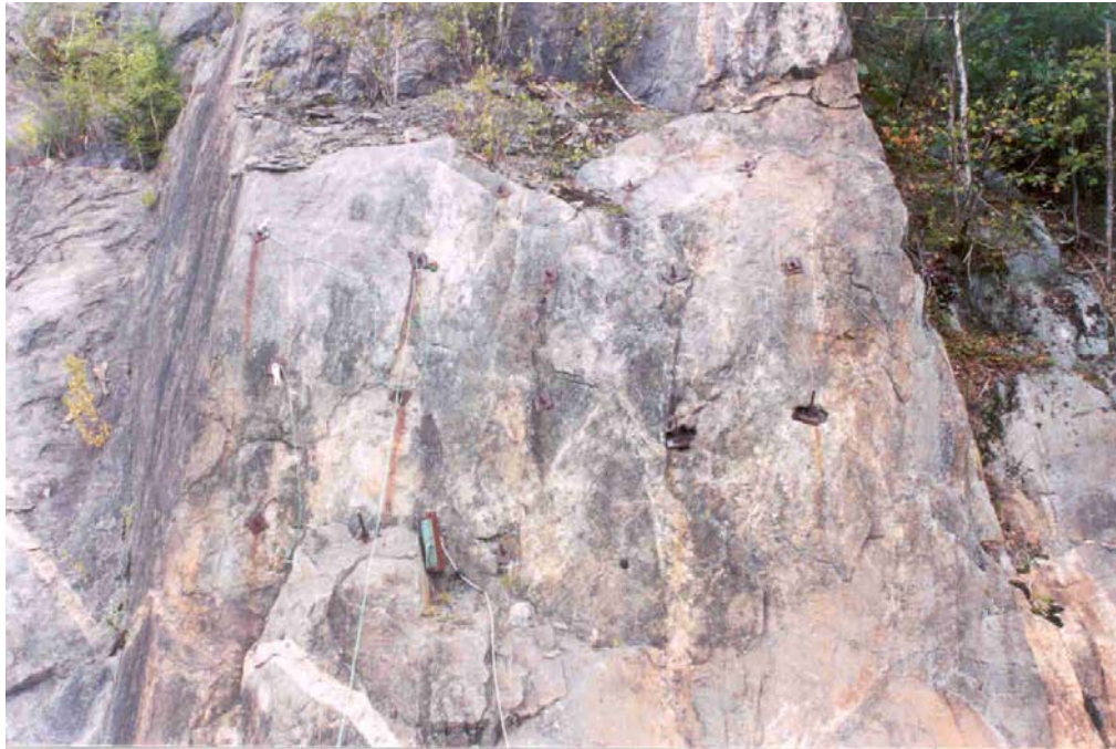
Photograph 11 – Half-cell location for Bolts 13 and 14. Half-cell was placed in a hole to the right of Bolts 13 and 14 (left center).
