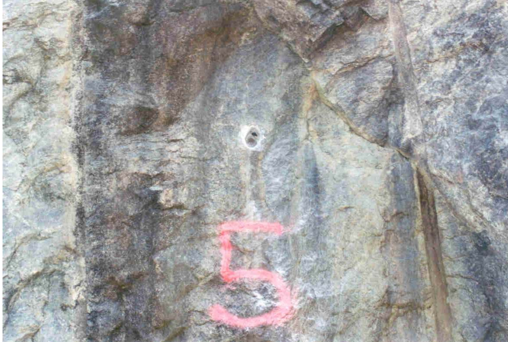
Photograph 9 – Exposed end of Tendon 5-2 after chipping
