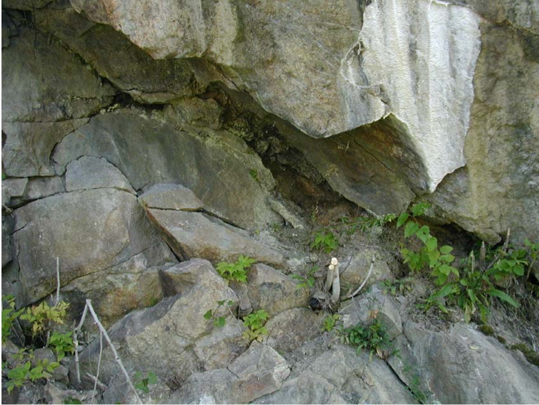
Figure 6. Weathered Rock Along Open Rock Joints
