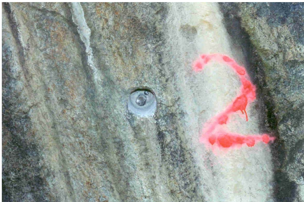
Photograph 2 – Exposed end of Tendon 2-1 after chipping
