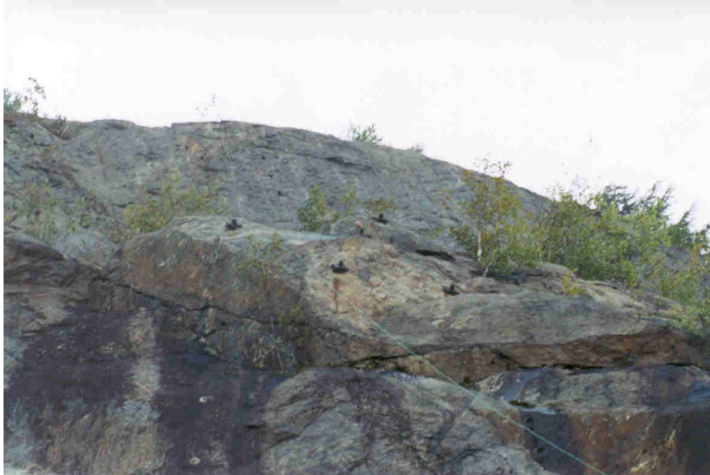
Photograph 15 - Half-cell location for Bolts 19 and 20. Half-cell was placed in the crack approximately 10 feet to the right of Bolt 20.
