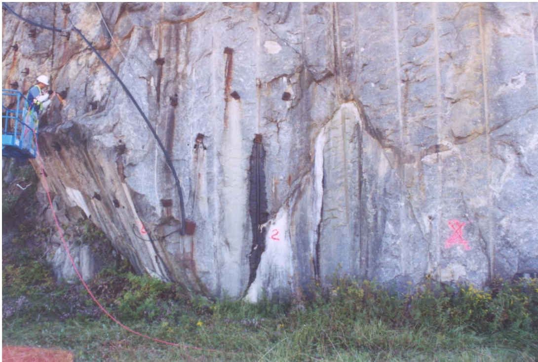
Figure 15. Leaching of Grout Near Tendon Sample 2-2.
