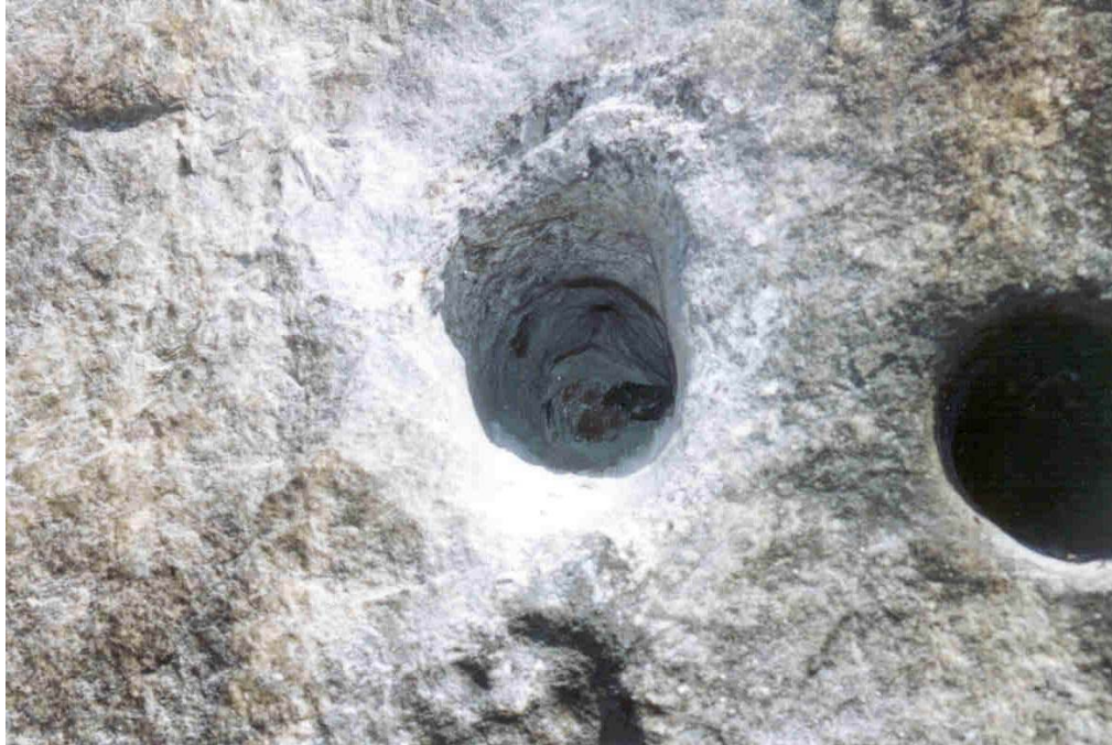
Photograph 1 – Exposed end of Tendon 1-1 after chipping
