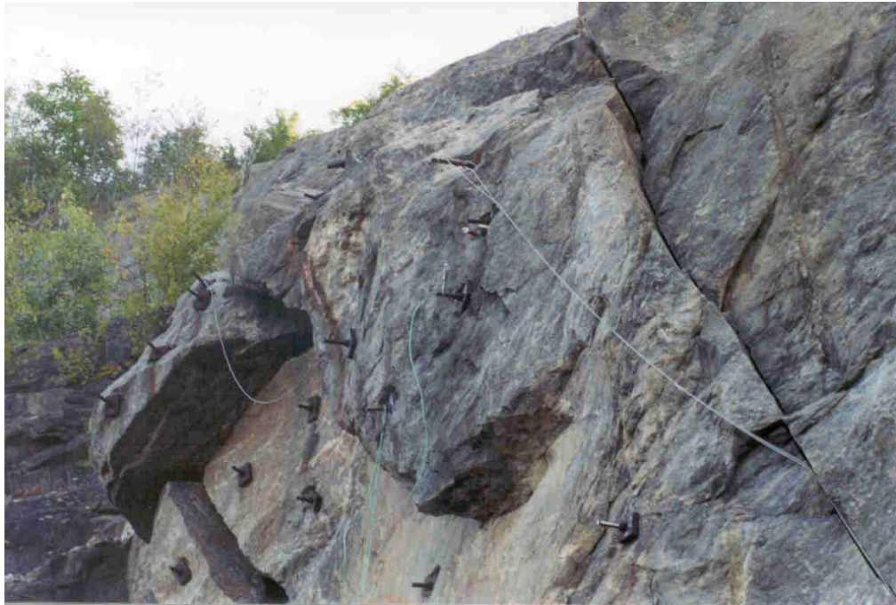
Photograph 9 – Half-cell location for Bolts 9 and 10. Half-cell was placed in a hole directly above Bolt 9 (center).
