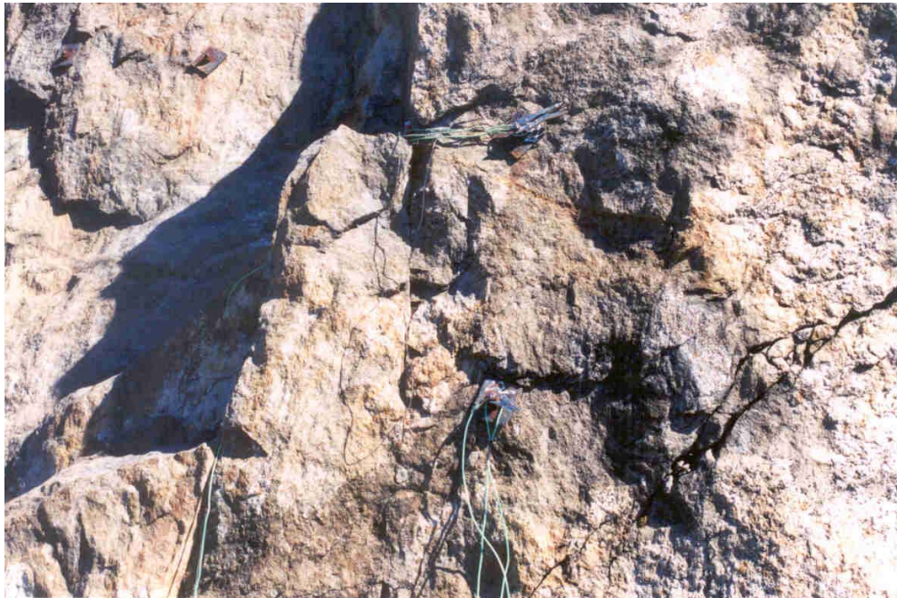
Photograph 16 – Half-cell location for Bolts 21 and 22. Half-cell was placed in the crack approximately 3 feet to the left of Bolt 21.
