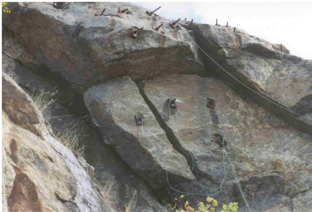
Photograph 12 – Half-cell location for Bolts 15 and 16. Half-cell was placed in the horizontal crevice, right of the near vertical crevice, in the center of the photo.
