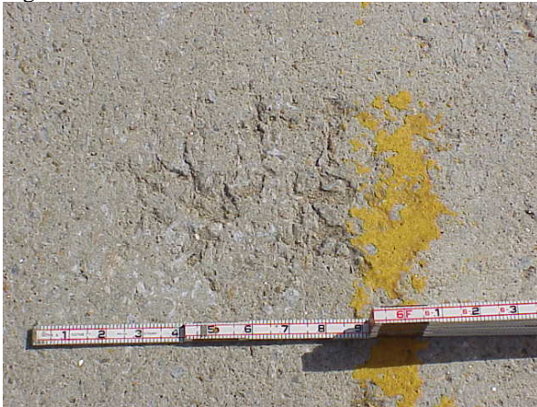
Figure 5: Centerline defect in fiber reinforced mix
