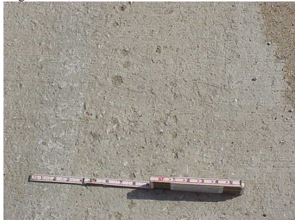
Figure 6: Shoulder defect in fiber reinforced mix
