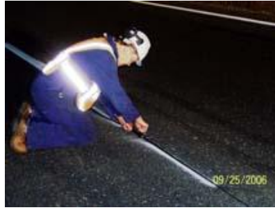
Backer foam is inserted over the tubing to protect it from crack sealant.
