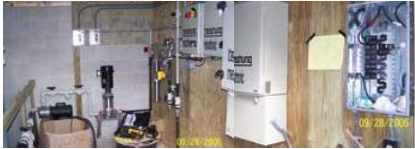
Pump house operational systems: pump, control valves and computer system (closed cabinets).
