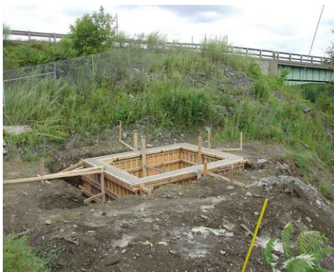
Cast-in-place concrete pump house foundation doubles as secondary containment for single-walled chemical storage tank.
