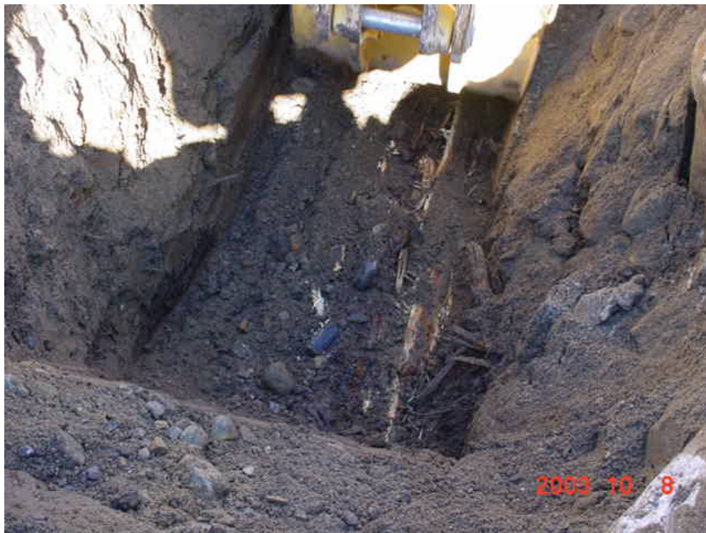
Figure 19: Test pit showing corduroy road.
