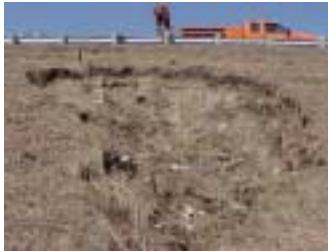
Figure 42: Embankment failure in Hudson, NH
