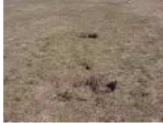
Figure 43: Voids on opposite side of road to embankment failure
