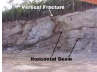
Figure 25: Horizontal seam and vertical fracture showing a detached slab
