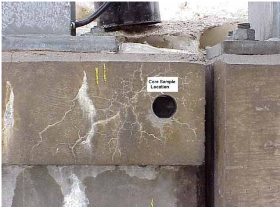
Photo 2 - Map cracking on facies, bridge over I-89 in Grantham, NH.
