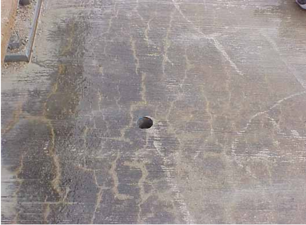
Photo 3 - Map cracking on sidewalk, bridge over I-89 in Grantham, NH.
