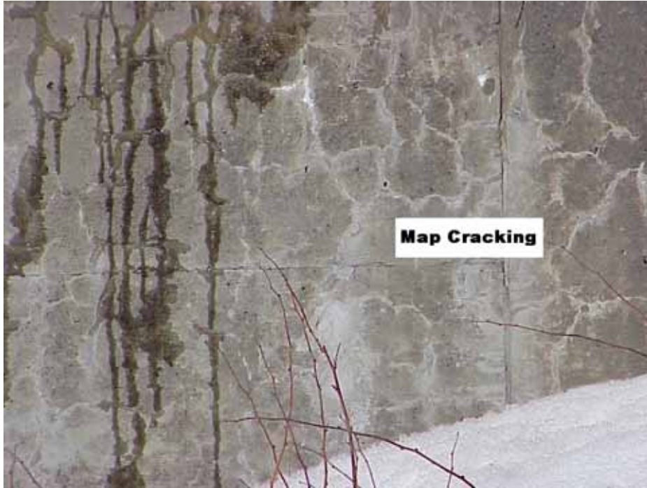
Photo 1 – Map cracking on wing wall, I-89 Northbound bridge over Frye Lane, Grantham, NH.
