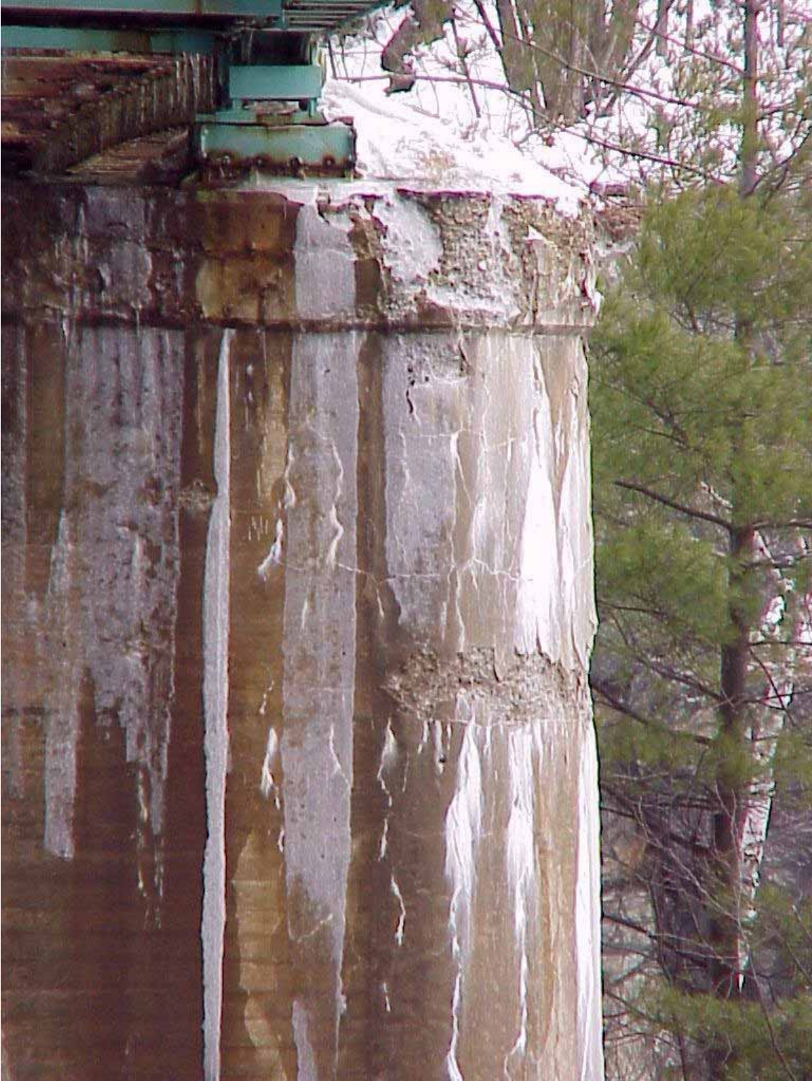
Photo 5 – Map cracking and deterioration of concrete on Connecticut River bridge pier in Monroe, NH.
