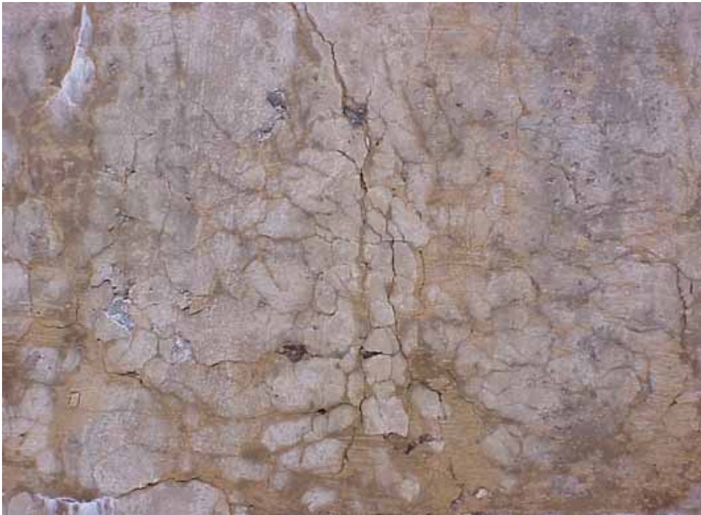
Photo 4 – Map cracking on bridge pier over Connecticut River in Monroe, NH.
