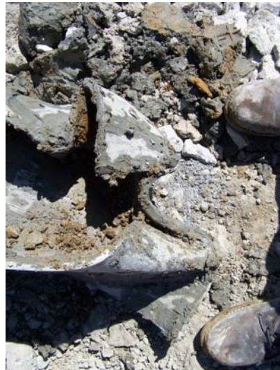
Pile P-Note web buckling
