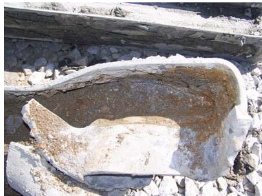
Missing teeth on Pile Point F web
