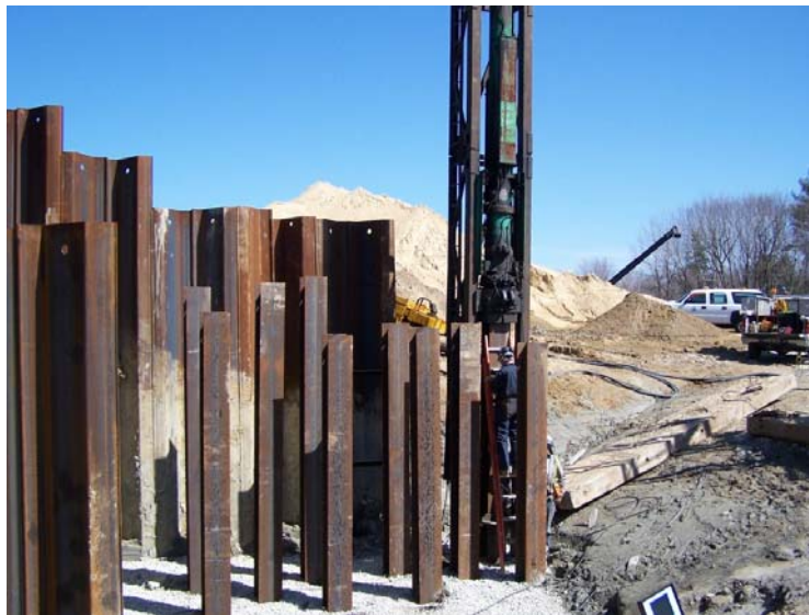
Test setup – Leads are on Pile G, sheet piles are retaining embankment
