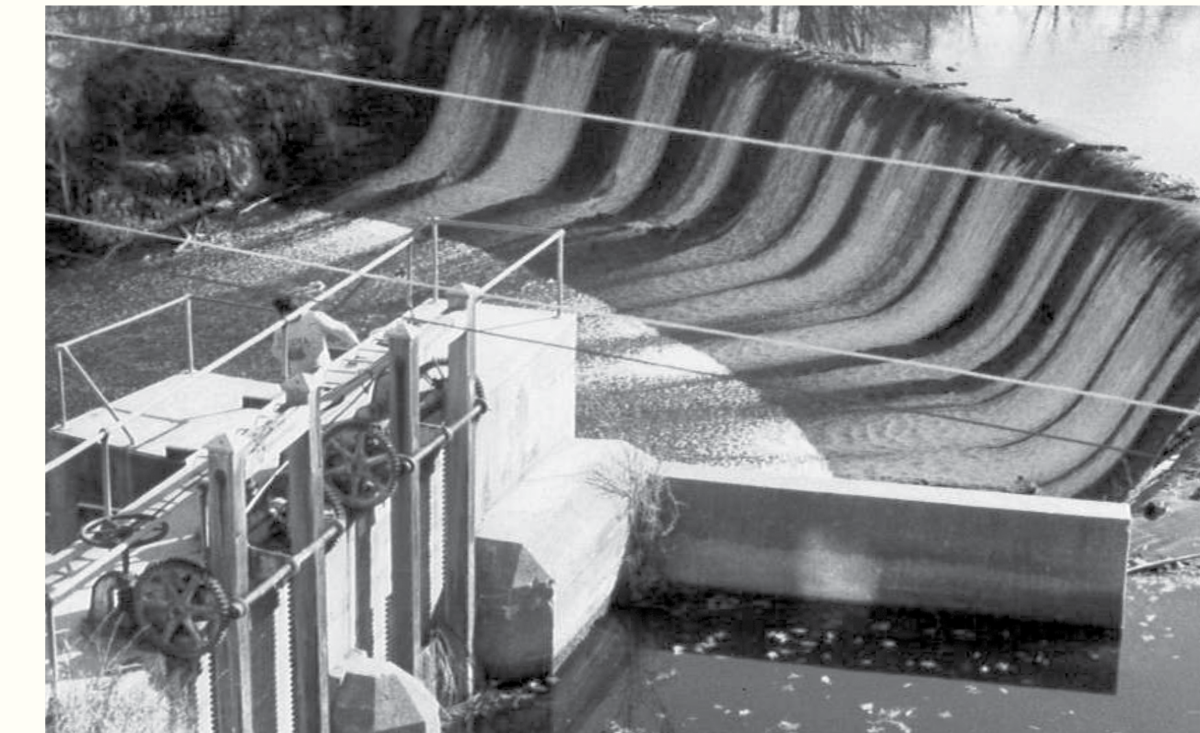
1989 photo of bridge, dam, and power canal head gate. The ogee design and continuation over the ledge eliminated water spray on the Chamberlain Bridge and passing cars. NH Dam Bureau
