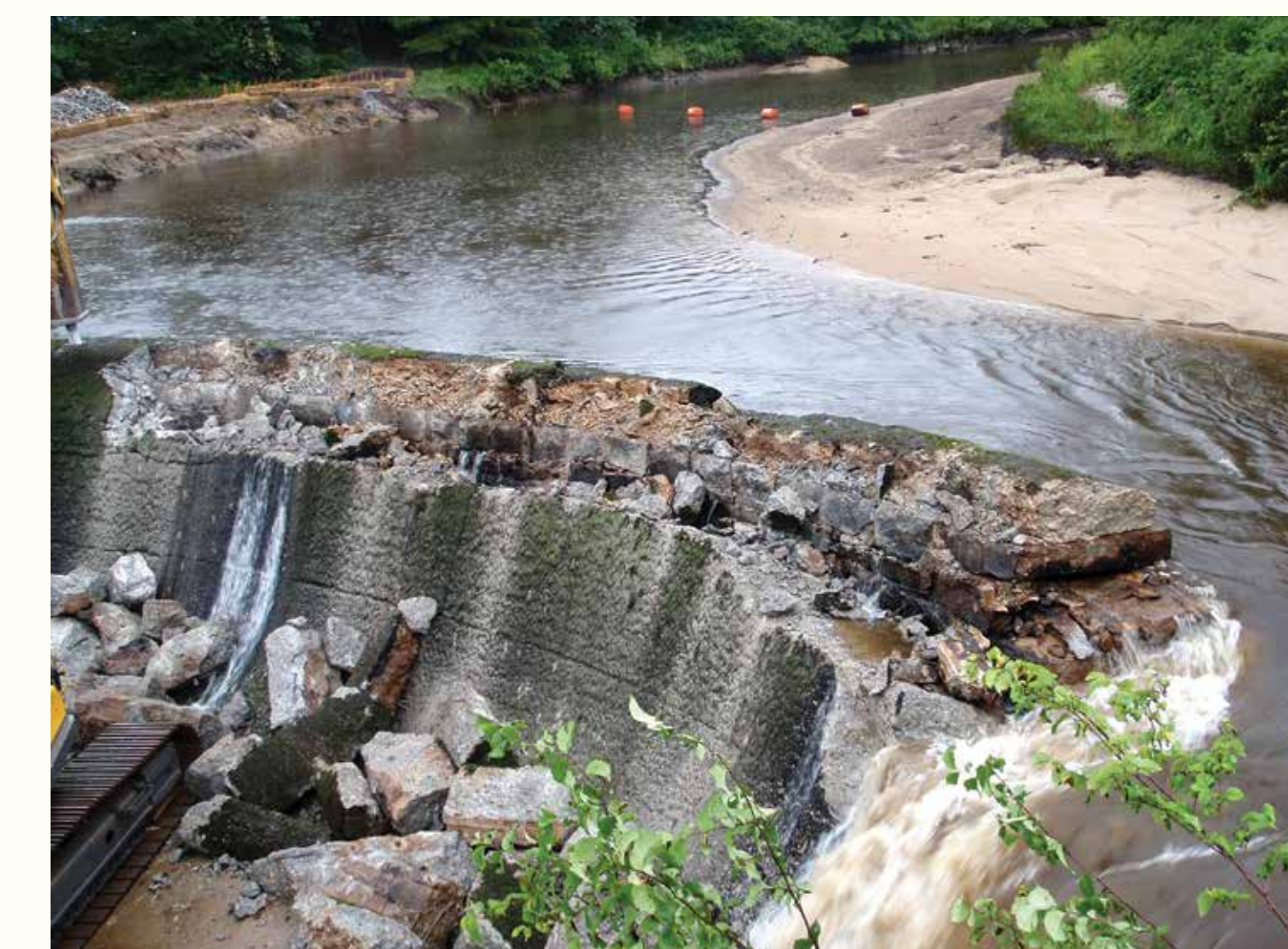
2008 photo of dam during demolition showing the rows of rectilinear, dressed, granite stones of the 1895 dam and thick layer of cyclopaean cement of the 1934 added ogee spillway. Mark Wamser
