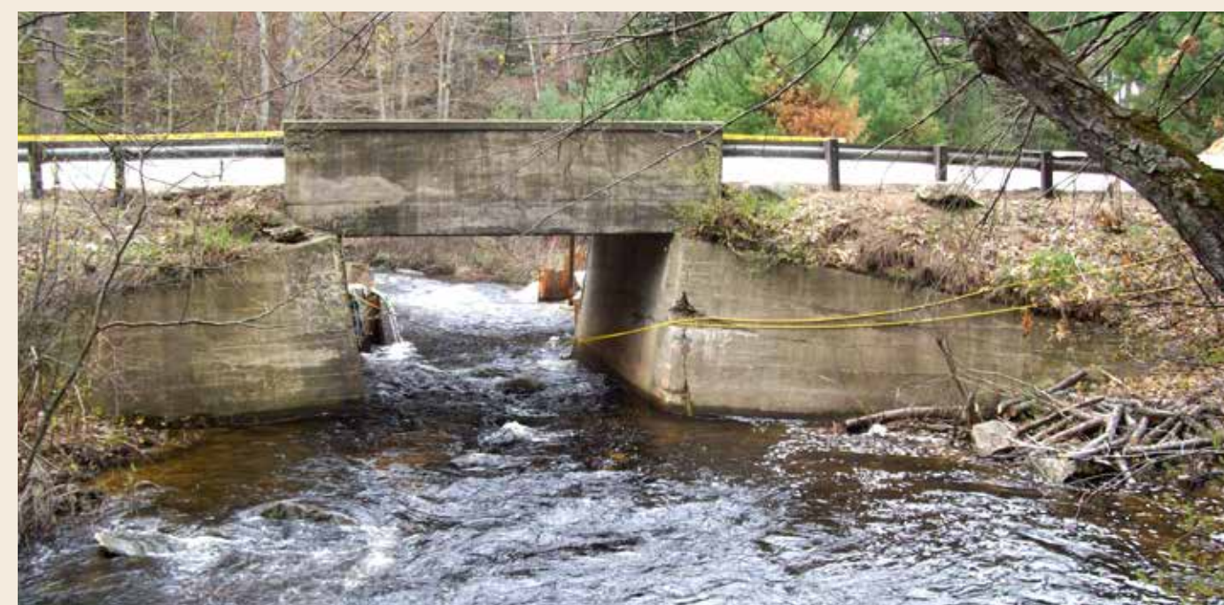
Robbins Bridge over Baboosic Brook before it was replaced in 2008. NorthEast Earth Mechanics
