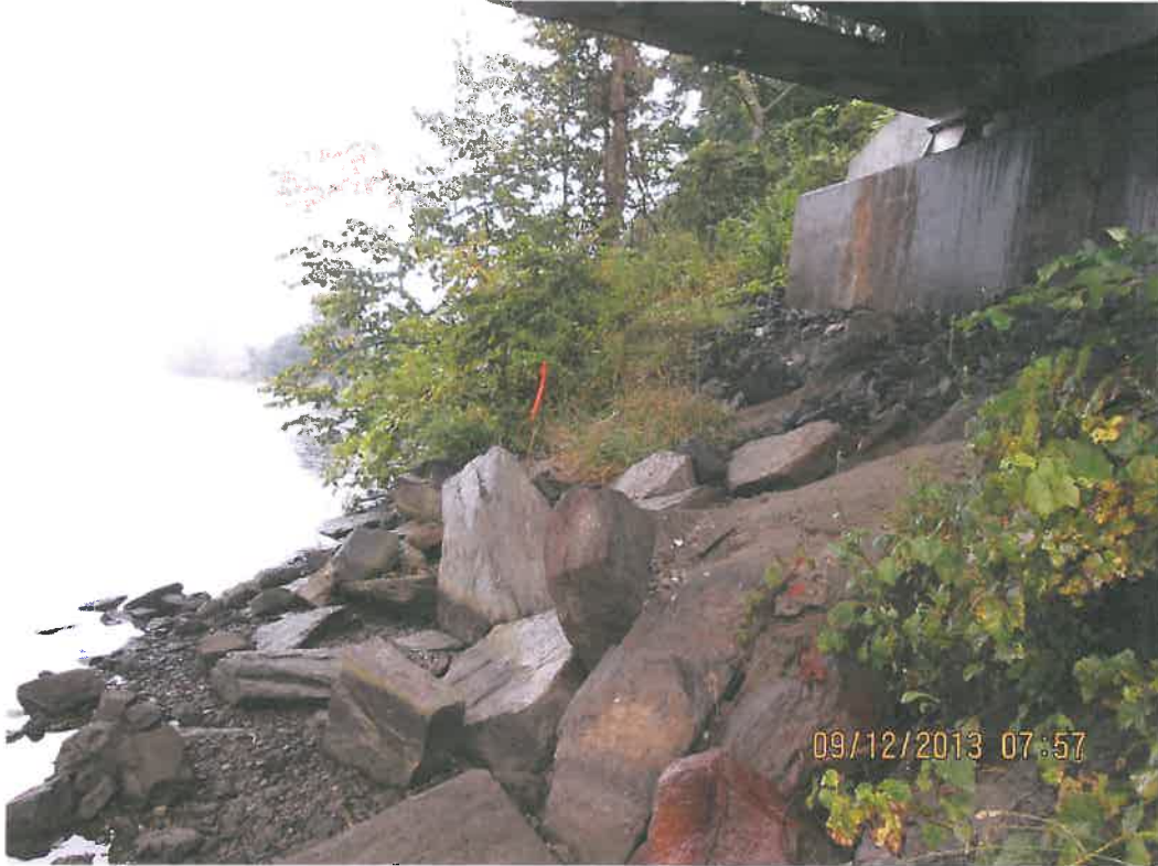
Photo 5 – View from NH shoreline looking northerly at existing river bank and bridge abutment to be temporary impacted to temporarily relocate bridge during pier replacement.
