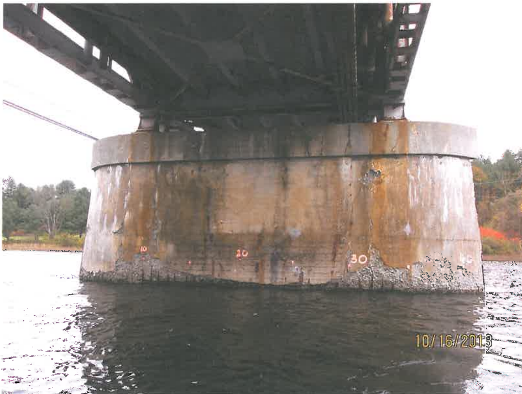
Photo 8 – Closeup view looking easterly at the VT side of the existing deteriorated pier.
