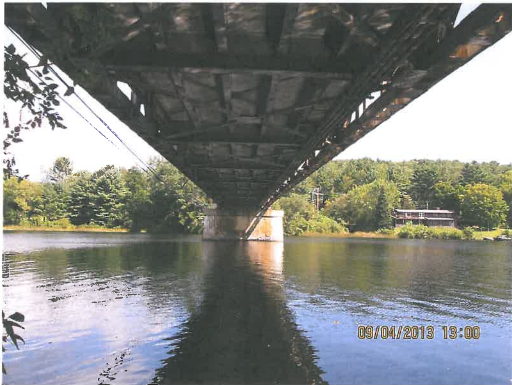
Photo 2 – View from VT shoreline looking easterly toward pier and NH shoreline at proposed areas of temporary trestles during reconstruction.
