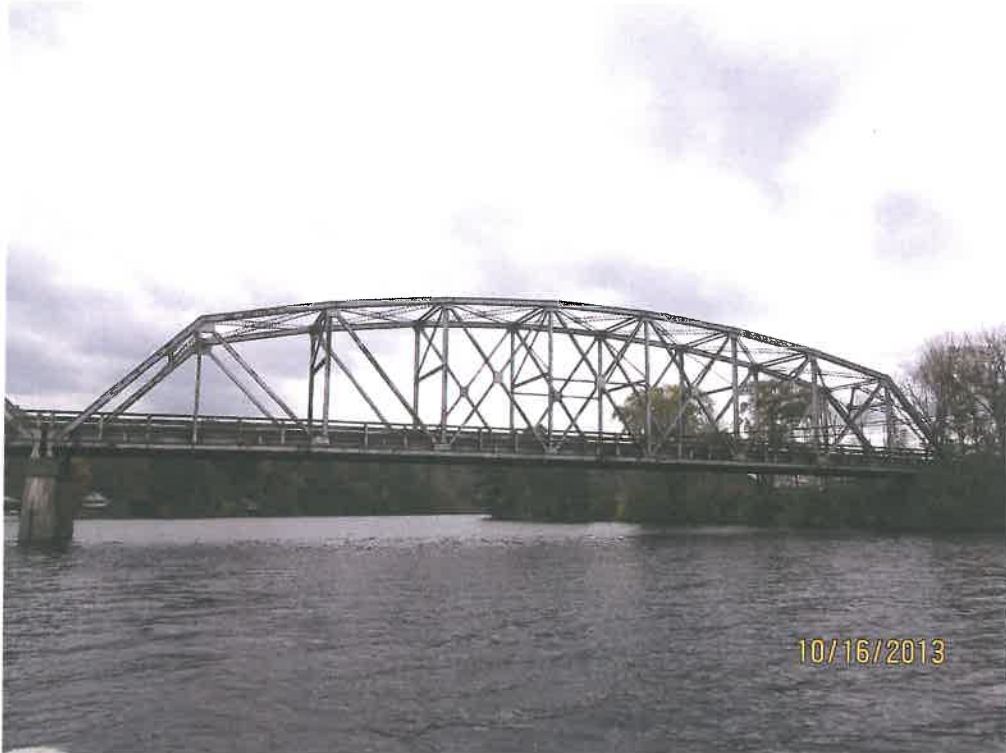
Photo 9 – View looking downstream of the westerly portion of the existing bridge and proposed area of temporary trestle during bridge and pier reconstruction located in NH and VT and temporary VT river bank impact for temporary bridge relocation.
