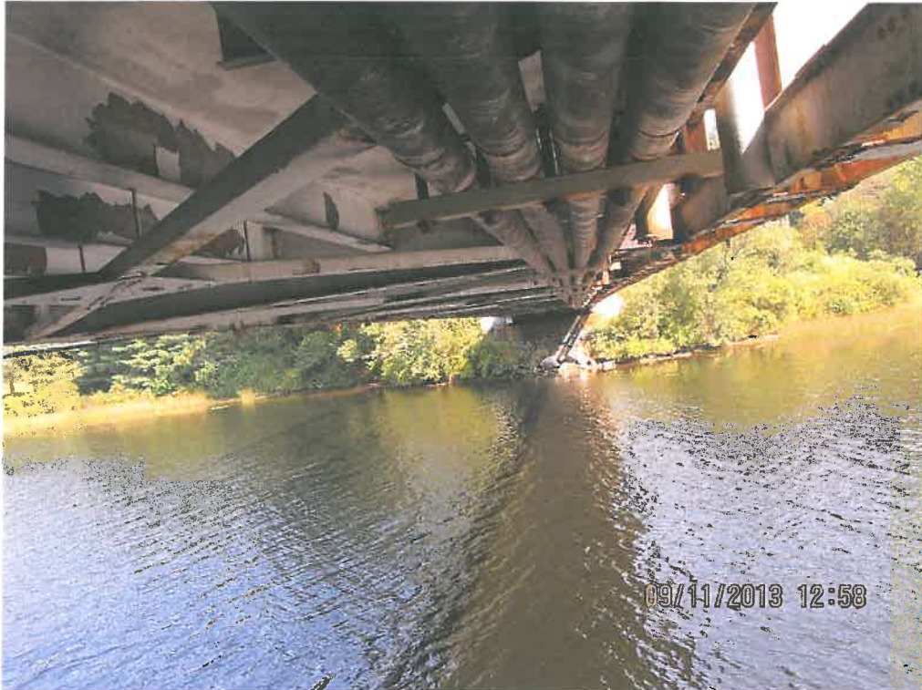
Photo 3 – View from top of existing bridge pier looking easterly toward NH shoreline and proposed temporary trestle location adjacent to pier and temporary bank impacts to relocate bridge during reconstruction.
