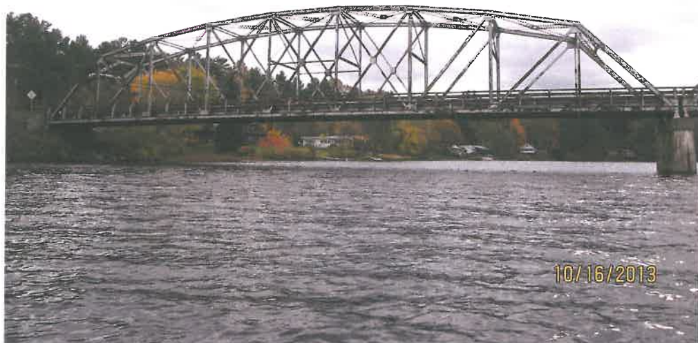
Photo 10 – View looking downstream of the easterly portion of the existing bridge and proposed area of temporary trestle adjacent to existing pier during pier reconstruction and temporary NH river bank impacts for temporary bridge relocation.
