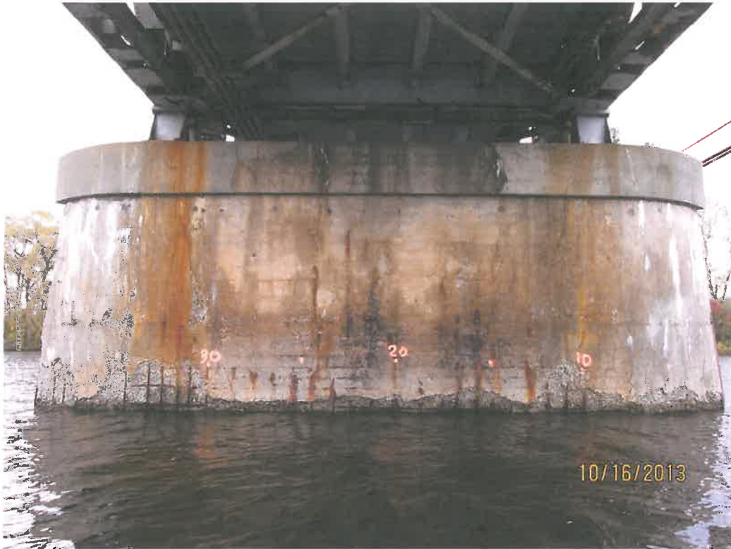
Photo 7 – Closeup view looking westerly at the NH Side of the existing deteriorated pier.
