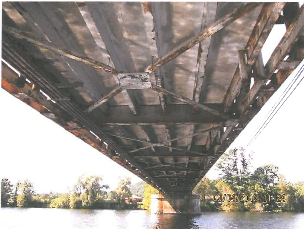
Photo 4 – View from NH shoreline westerly toward VT shoreline of area of proposed temporary trestle location and access from VT. VT access to be in shoreline tree line gap seen in lower left of photo.
