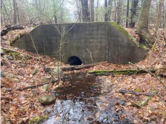
Photo 5. The outlet of Pool 1 Photo taken 8 April 2022.
