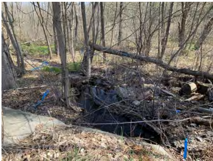
Photo 11. Facing downstream above the 24" RCP carrying Stream 2 under the intersection of Stonehenge and Rockingham Road.
