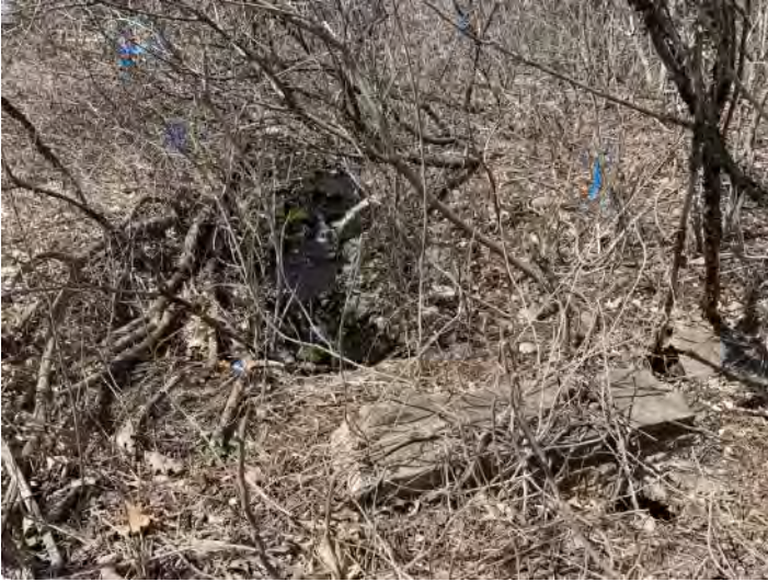
Photo 13. Facing upstream above the 24” culvert carrying Stream 2 under the intersection of Stonehenge and Rockingham Road.
