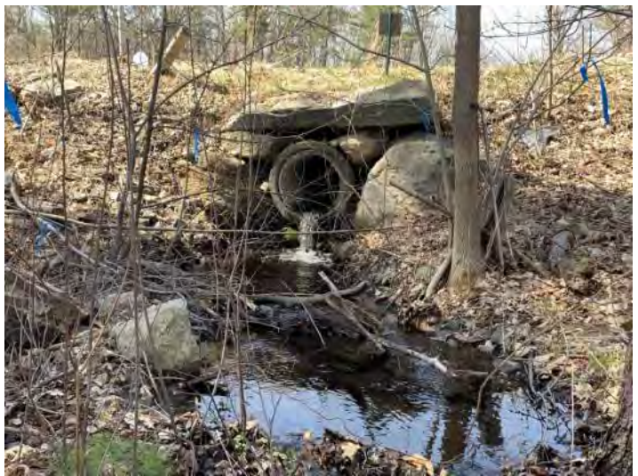
Photo 12. The outlet of the culvert carrying Stream 2 is perched by approximately 1.5 feet.
