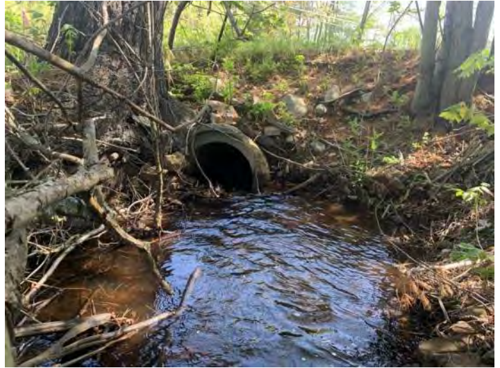
Photo 18. The headwall of the inlet of Stream 1 is deteriorated. (*photo taken 17 May 2022).
