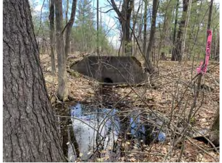
Photo 2. Wetland A is modified by an old woods road culvert that carries flow from the wetland through NJDA-1 to Wetland D.
