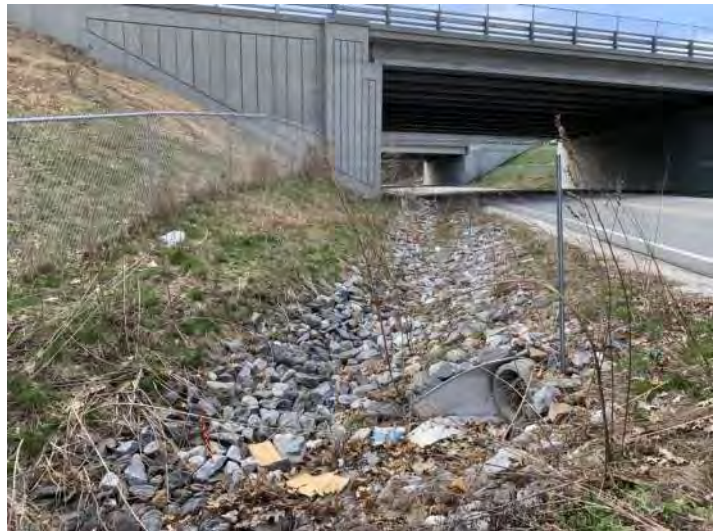
Photo 16. NJDA-2 is a stone swale carrying stormwater runoff from Stonehenge Road to Stream 1.
