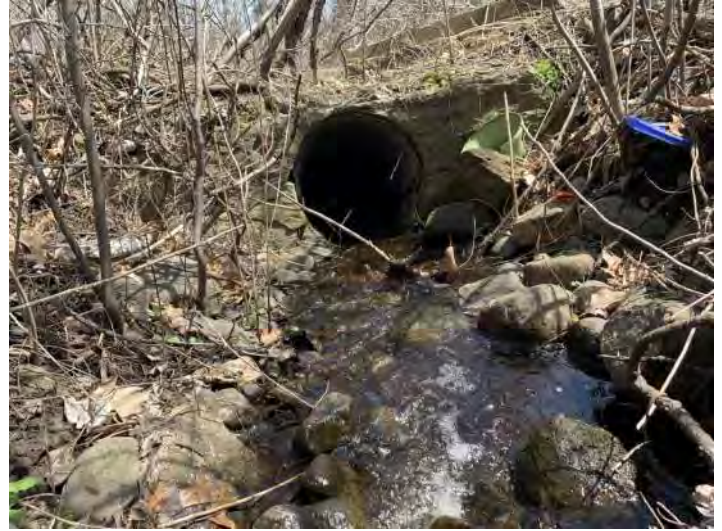
Photo 14. Stream 2 flowing into the inlet of the crossing. The headwall and culvert are deteriorating.
