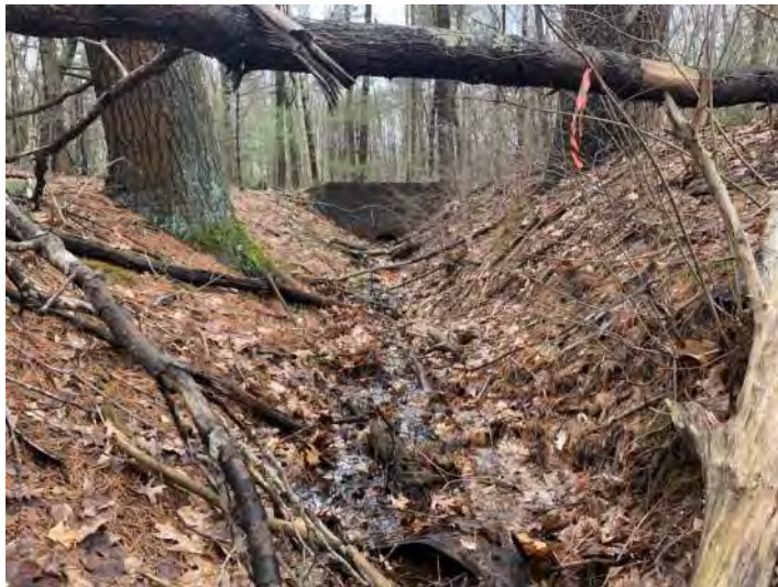
Photo 3. NJDA-1 connects Wetland A to Wetland D through a series of culverts. (*Photo taken 9 April 2022).
