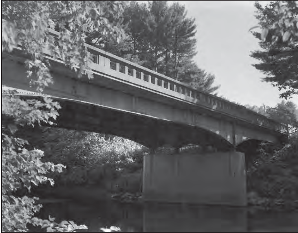
Figure 9. Winchester-Swanzey Bridge, Oblique View of Bridge's Western Elevation, Looking South. September 2013 (Photograph by David Haas in Harshbarger, "Winchester-Swanzey Bridge," 2013).
