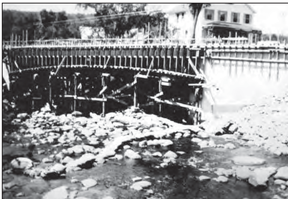
Figure 7. Construction of the N.H. Route 11 over Backwater River Bridge, Town of Andover (State Bridge No. 053/092). Circa 1934. This photograph shows the falsework in place (Whittum Family Papers).
