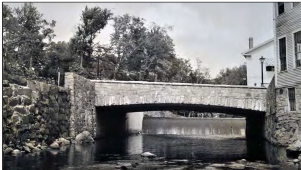
Figure 13. Grove Street over the Nubanusit River, Town of Peterborough. State Bridge No. 087/087. Circa 1936. Design by Gordon R. Whittum (NHDOT Bridge Card).
