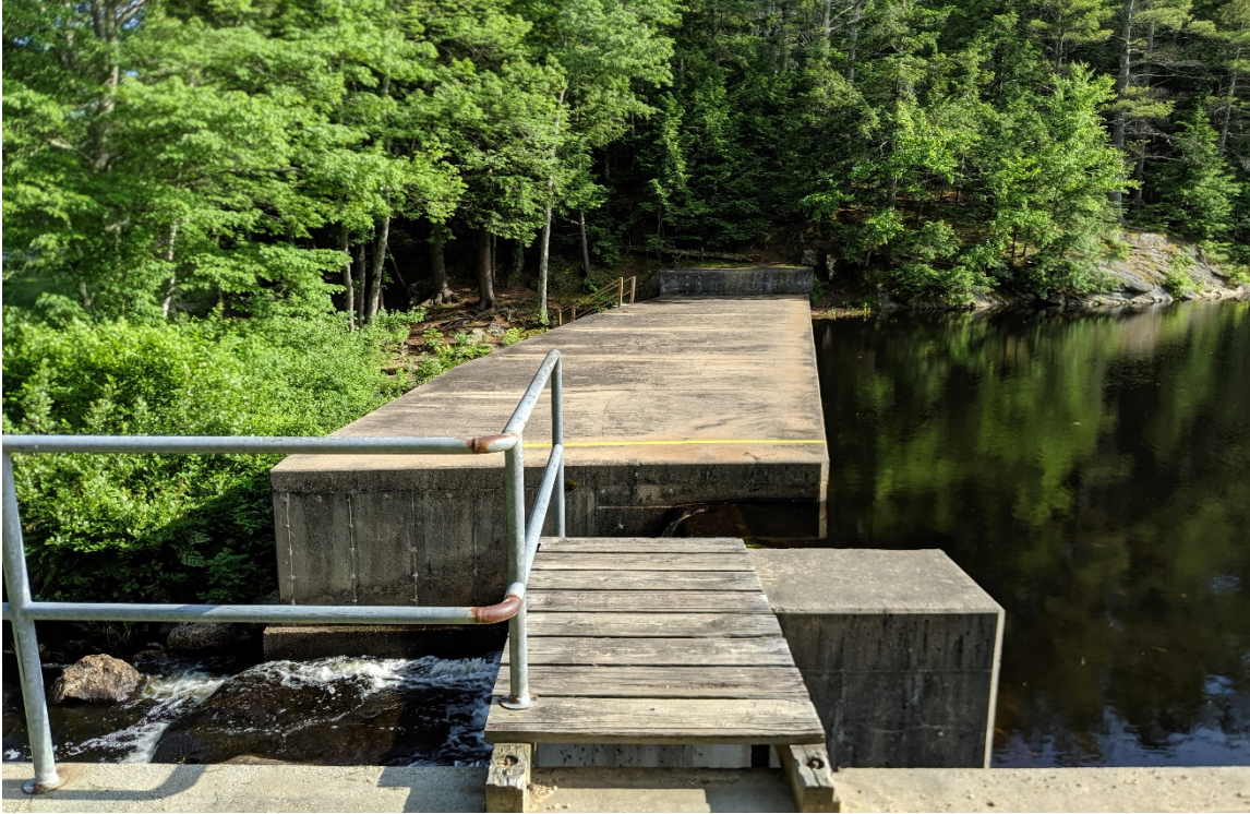
Photo 13: View south of the Freeses Pond Dam that impounds the Lamprey River (6/27/19).
