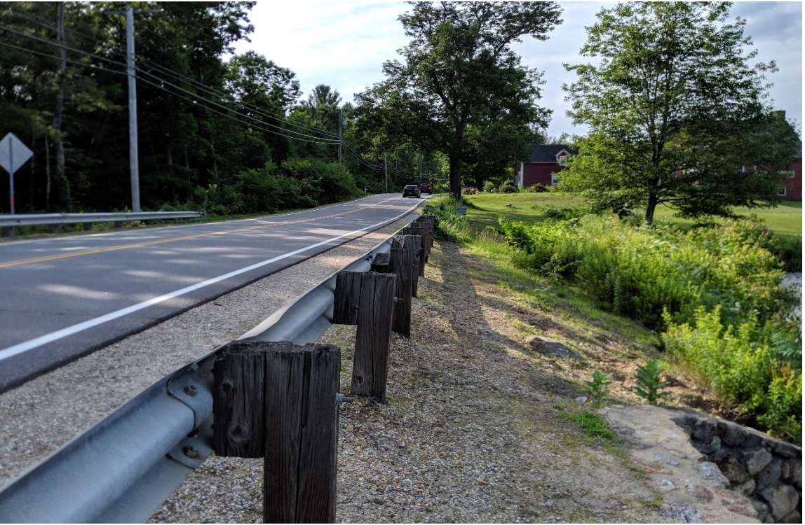
Photo 2: View northeast of NH 107 within the proposed project area, taken from the upstream side (6/27/19).
