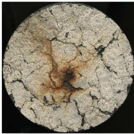
Figure 1 Concord core showing source of major iron staining
