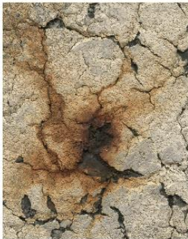
Figure 2 Close up of Figure 1 showing iron staining
