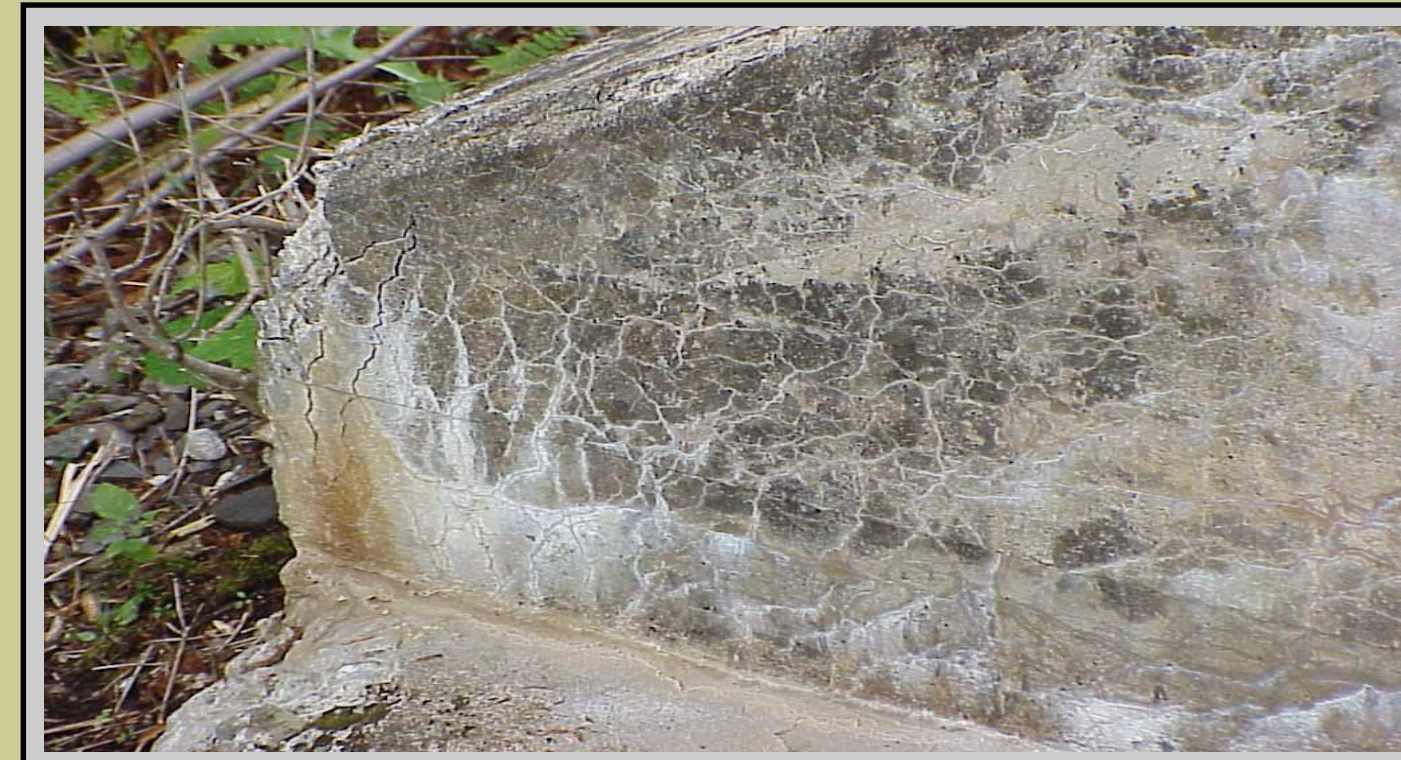
White precipitate exuding from map cracking of abutment wing wall, Frankenstein Trestle, Crawford Notch
