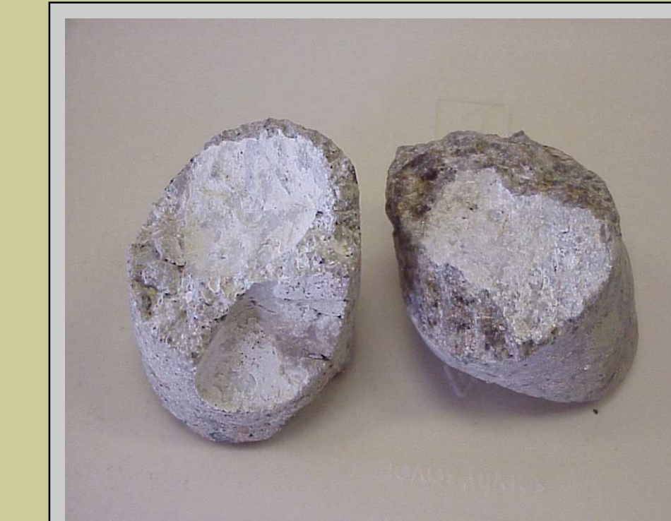
White precipitate lining pop-outs Swimming Hole Bridge, Woodstock
