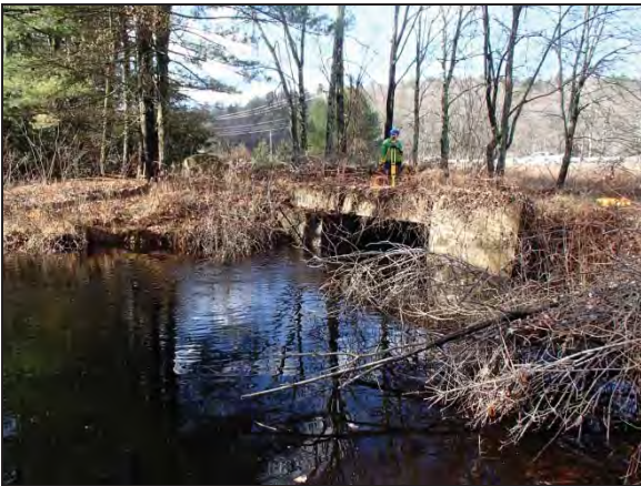
View upstream and across Pulpit Brook at outlet of abandoned bridge. Photo date: 12-01-16
