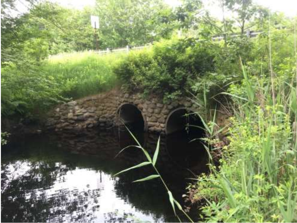
Photo 5, above. The downstream face of the existing twin culvert at the Pulpit Brook crossing. 6/16/17. (Temporary impacts K, L, M, and N, and permanent impacts G, H, I, O and Q at this location)
