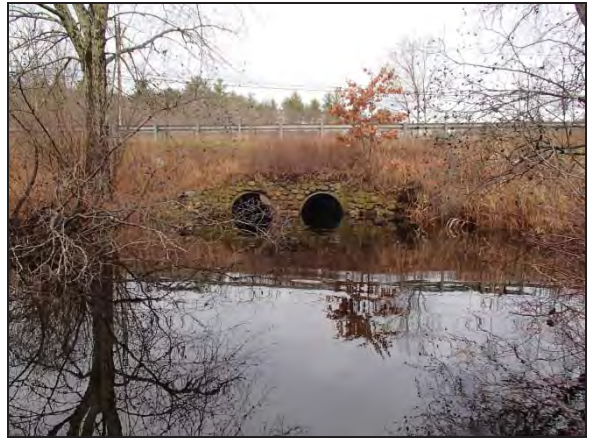
View upstream at outlet of existing twin 60" RCP culverts carrying Pulpit Brook under Route 101. Photo date: 12-01-16
