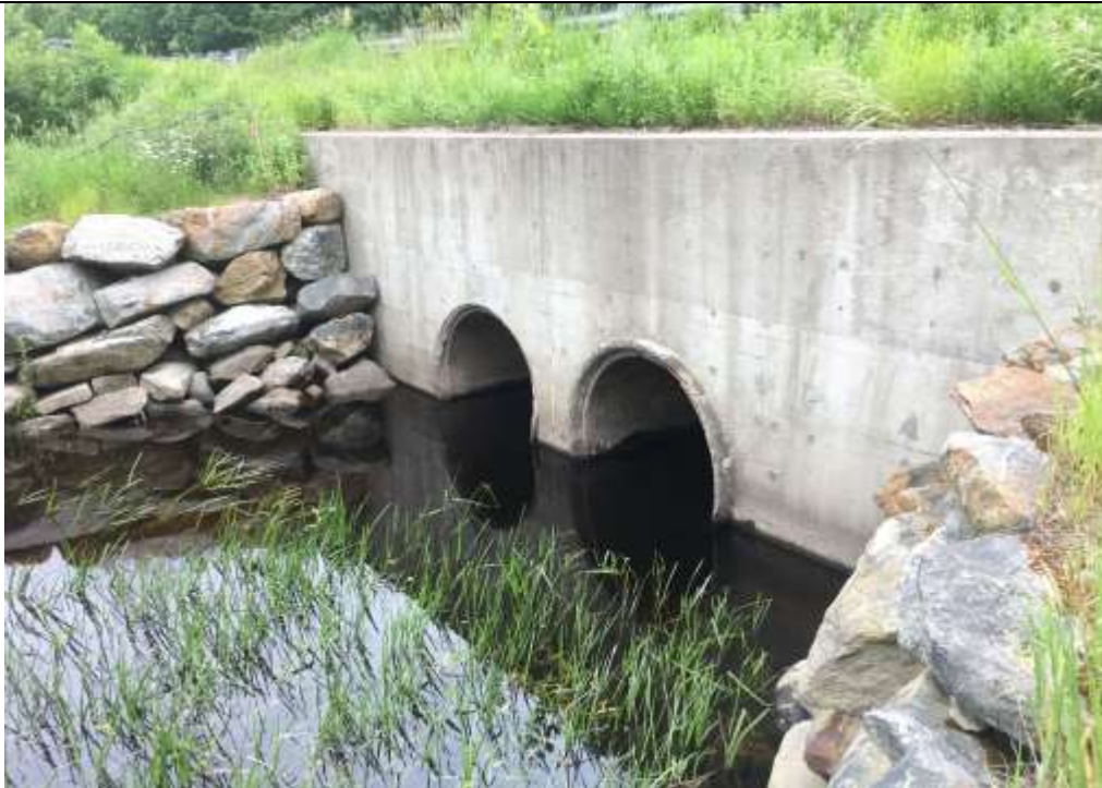
Photo 6, below. The upstream face of the existing culverts. 6/16/17. (Temporary impacts B, D, and F and permanent impacts A, C, and E at this location)
