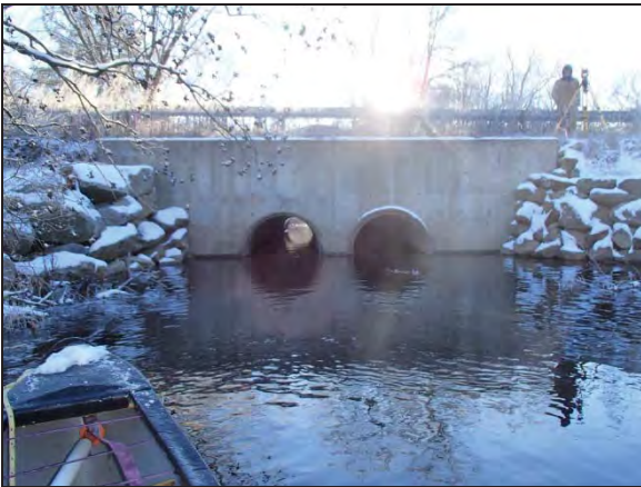
View downstream at inlet of existing twin 60" RCP culverts carrying Pulpit Brook under Route 101. Photo date: 12-06-16
